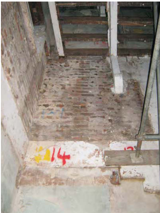
Plate 3: The exposed ground floor fabric of the west end of the north wall
