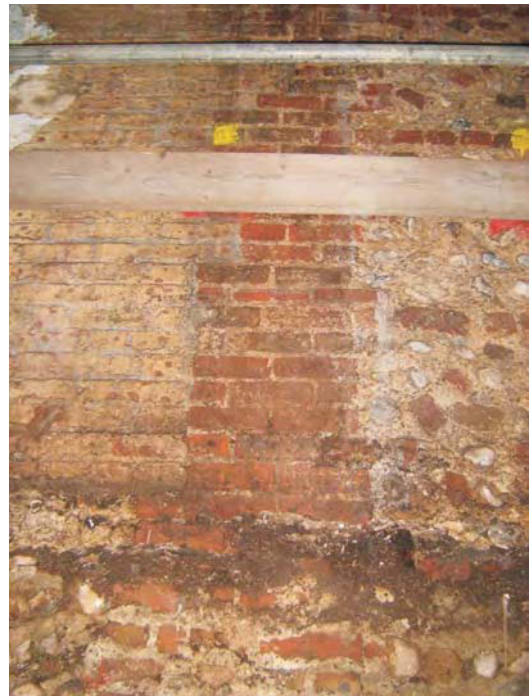
Plate 7 : The continuation of the brick pier to ground floor fabric in the east end of the north wall
