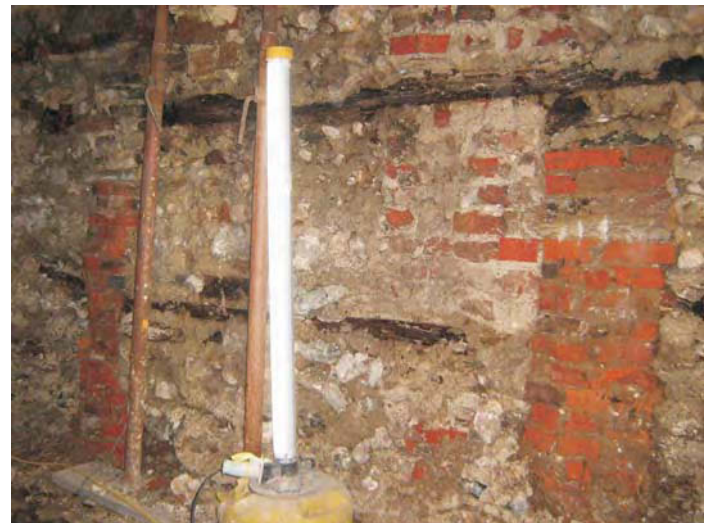
Plate 4: The north wall to the east of the modern entrance showing the timbers and the truncated red brick features
