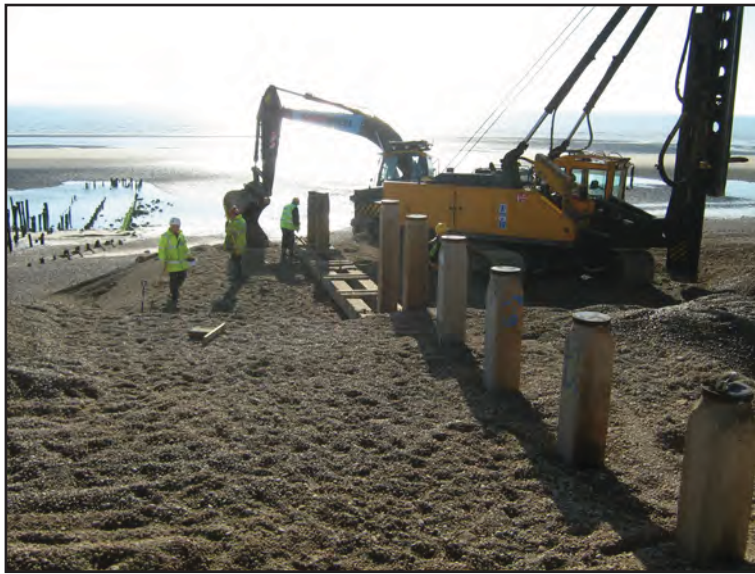
Figure 9: Work on Groyne W6 in progress, showing East Pier to left of shot
