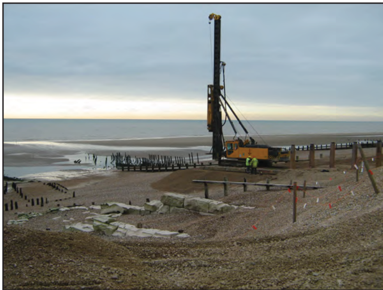
Figure 10: Work on Groyne W6 in progress, showing East Pier and West Pier
