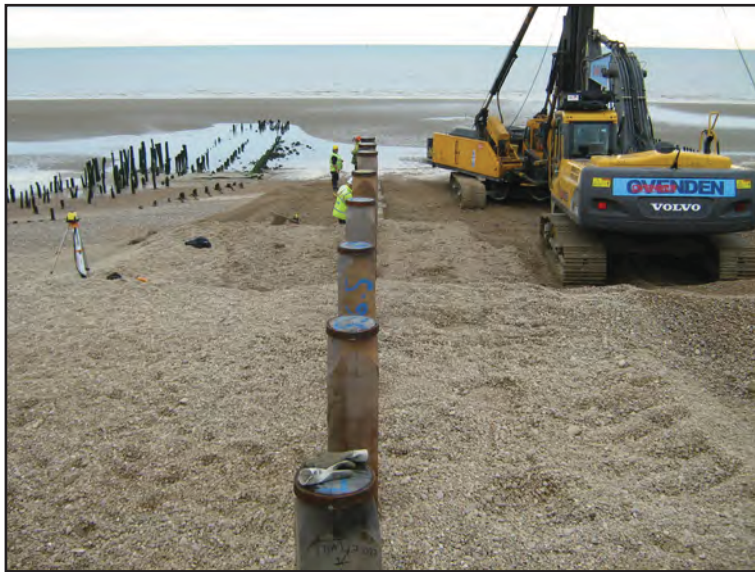
Figure 11: Work on Groyne W6 in progress, showing East Pier to left of shot
