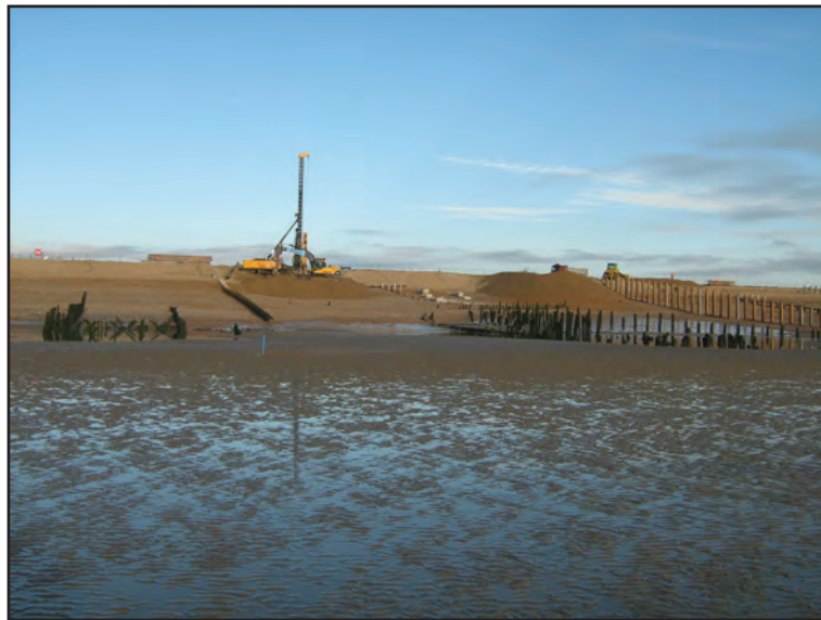
Figure 7: Piling on Groyne W6, showing West Pier to left and East Pier to right
