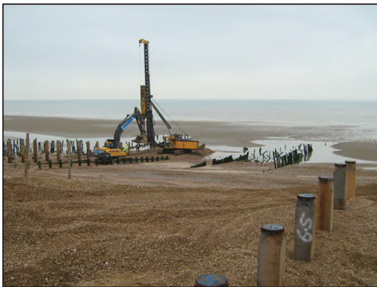
Figure 13: Work on Groyne W6 in progress, showing the start of Groyne W5
