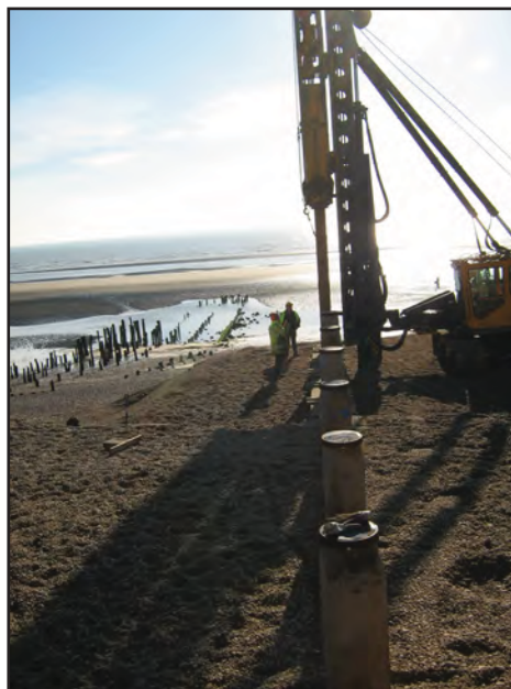
Figure 8: Piling on Groyne W6 in progress, showing East Pier to left of shot
