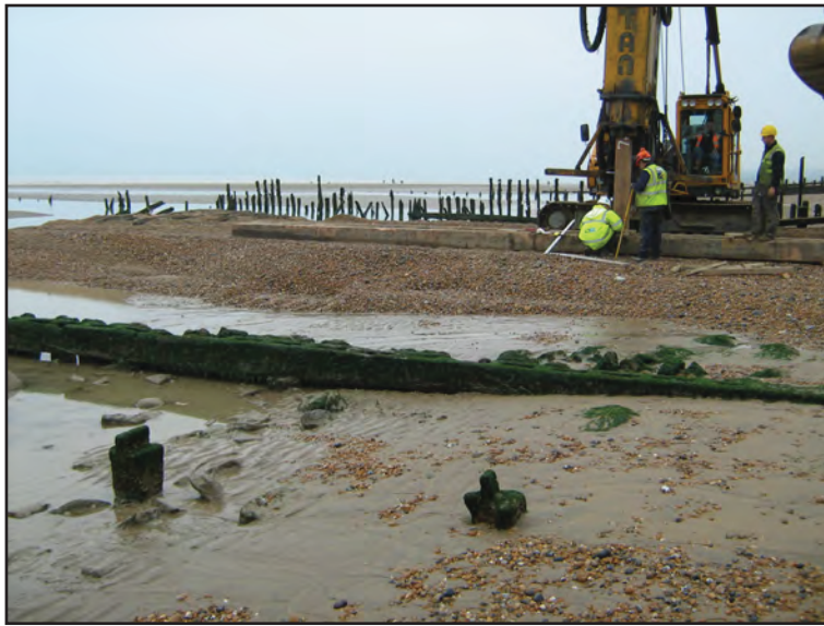
Figure 12: Work on Groyne W6 in progress, showing East Pier and West Pier
