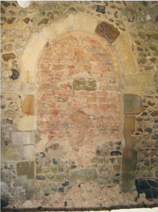
Figure 8: The un-blocking in progress showing the brick skin behind the outer face of flint.
