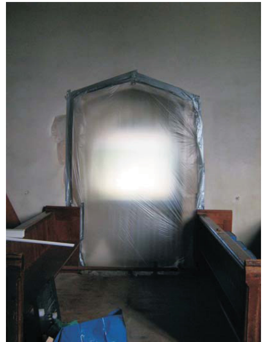
Figure 5: Interior view of the doorway, protected by plastic, but with the outline of the four centred arch visible
