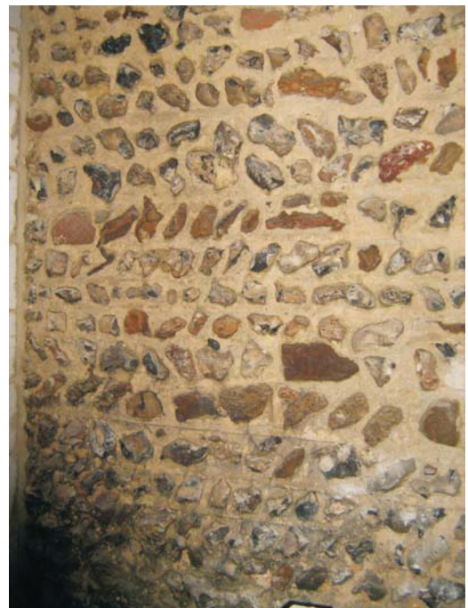
Figure 7: Detail of the fabric of the north wall to the east of the doorway
