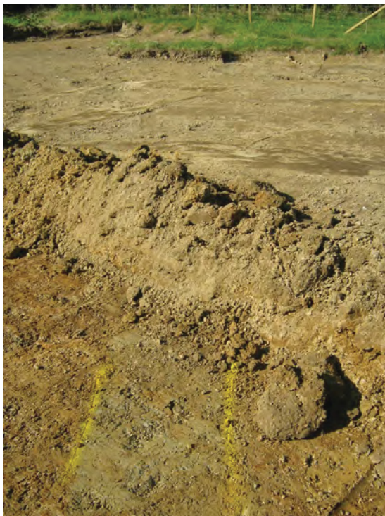
Fig. 4: North-west facing shot showing modern trench in foreground, with manhole MH8702 in background
