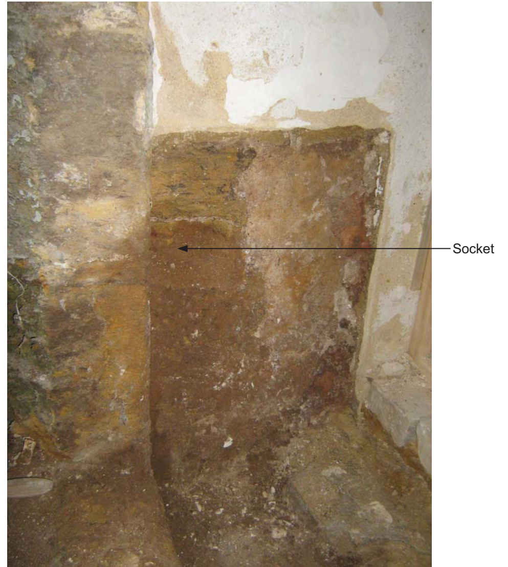
Fig. 10: The socket at the base of the west side of the doorway
