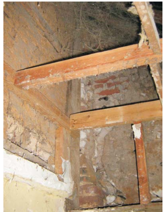
Plate 12: The east end wall of the outshot shows much modification and patching to the construction
