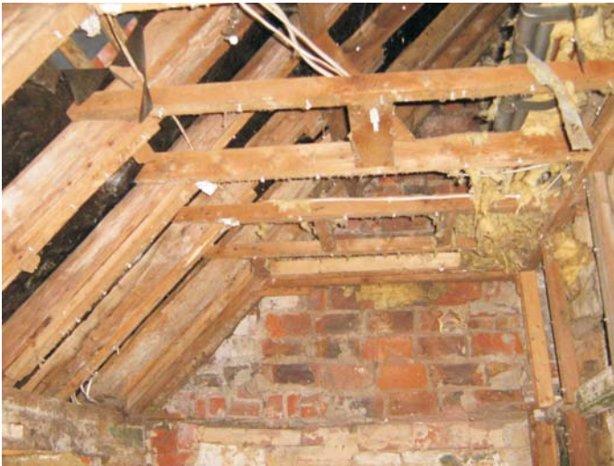
Plate 15: The construction of the west wall of the outshot with brick laid on edge above the off-set. The added softwood struts for the inserted under-plastered ceiling are also visible
