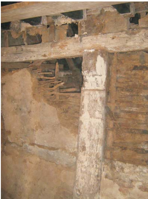
Plate 3: Detail of the two types of in-fill on the south partition wall of the living room
