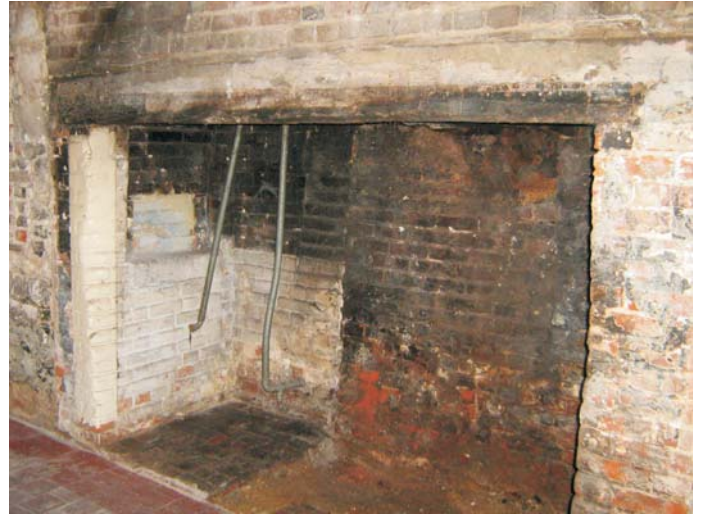
Plate 41: The south side of the inglenook with probable bread oven which had been hidden by the added south cupboard
