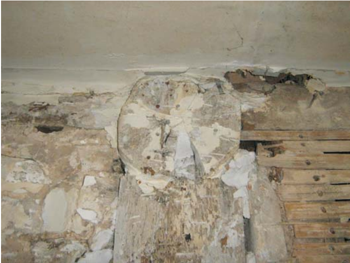
Plate 48: Timber plate at the top of the post in the north wall of the former kitchen
