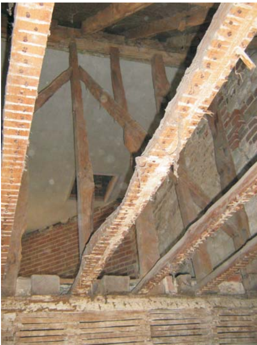
Plate 50: The timber frame south wall of bedroom 2 viewed through the removed ceiling of the former toilet. The view shows substantial joists over the side girt, and the softwood timbers of the under-plastered ceiling
