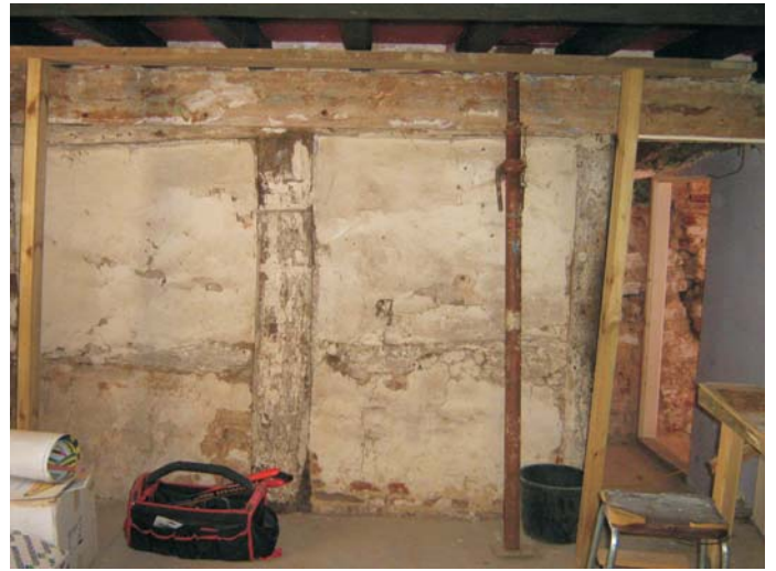
Plate 2: The small-panel framing in the south partition wall of the living room
