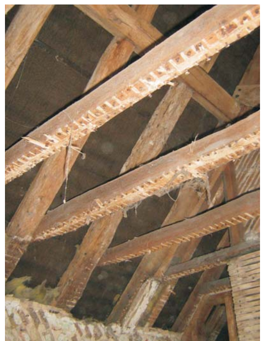
Plate 51: The roof construction of the outshot at the east end of the house
