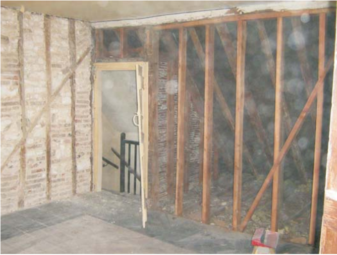
Plate 64: The later softwood construction of the south timber framed wall of bedroom 1
