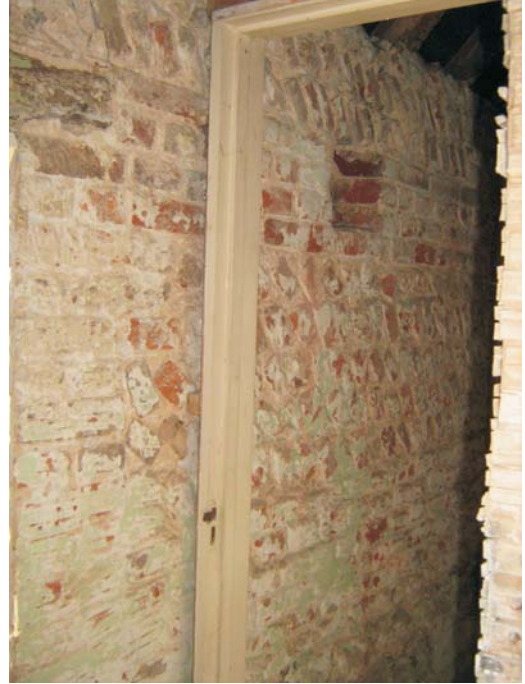
Plate 49: The south wall of the outshot - shows the herringbone brickwork at the top of the wall viewed from the interior of the former bathroom
