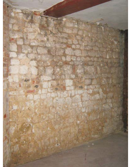
Plate 43: The east wall to the south of the fireplace shows the three blocked features which may have been storage recesses
