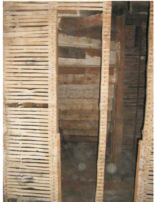
Plate 53: The underside of the staircase and the laths over the stud work viewed from the interior of the bathroom
