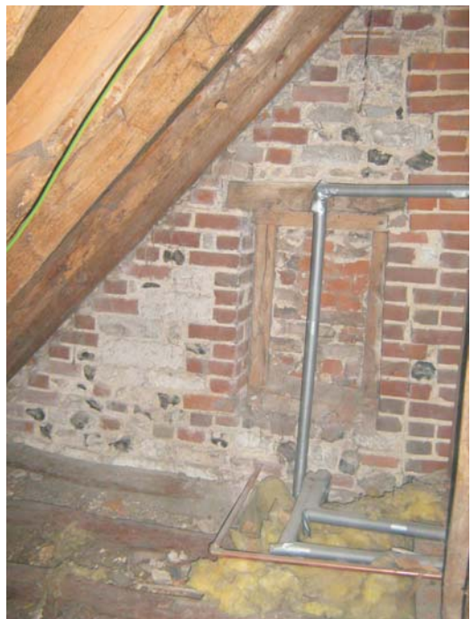
Plate 63: the blocked window in the west wall of the outshot in bedroom 1
