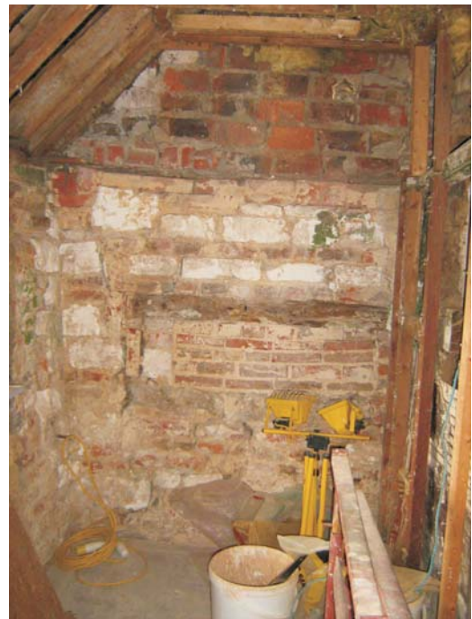
Plate 16: The lower chalk and brick built west wall of the outshot- with timber lintel and blocked feature/ recess
