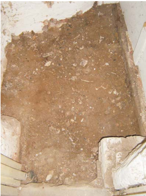
Plate 23: The floor after the removal of the softwood framework which had supported the boards
