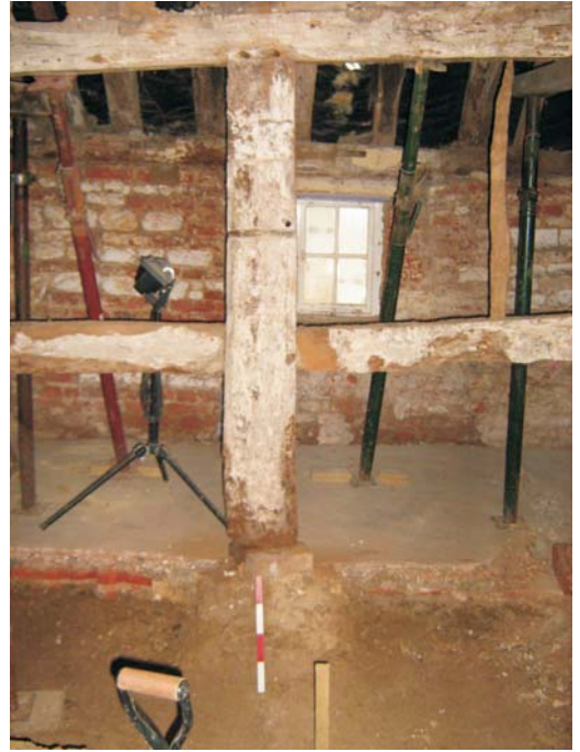
Plate 6: The full stripped wall with brick floor below the concrete in the former bathroom beyond
