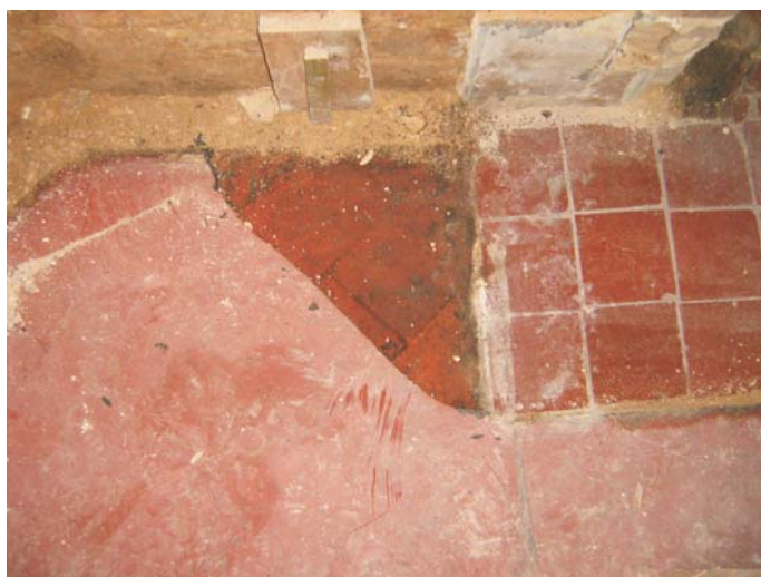
Plate 47: The sitting room - detail of the floor underlying the concrete screed adjacent to the fireplace
