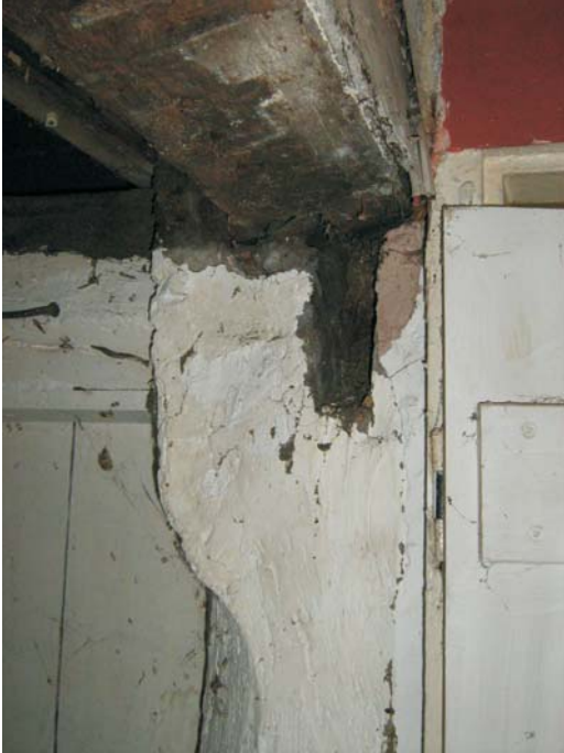
Plate 21: The post of the timber frame, within the cupboard to the south of the kitchen inglenook. There is a redundant mortise where the bressumer would have terminated prior to truncation caused by the insertion of the cupboard
