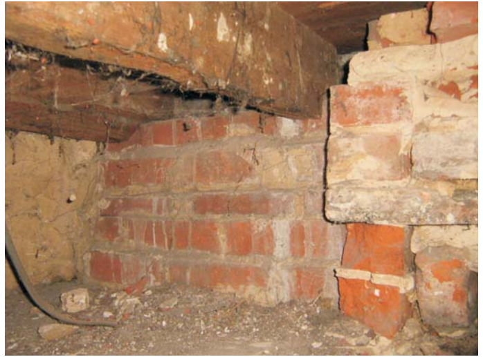
Plate 14: The modern brick inserted over the oven to support the stair construction - viewed from the living room side
