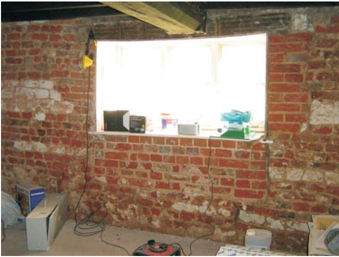
Plate 1: The east wall of the living room with the late phase of brick in-fill to a former, much larger opening
