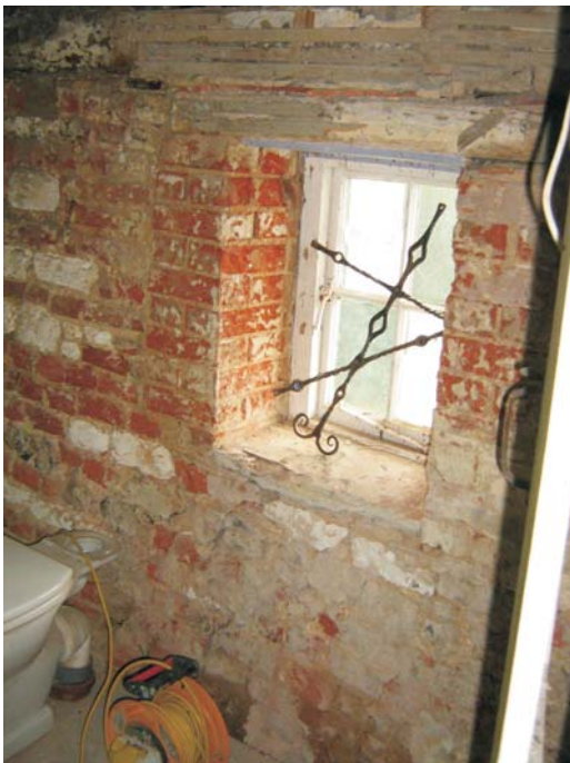
Plate 11: The 19th C bathroom window in the south wall of the room within the chalk block and brick built fabric of the wall
