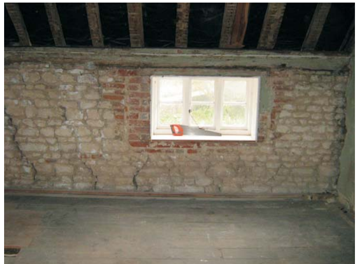
Plate 24: The north wall of Bedroom 1 shows 19th century casement within reduced original opening
