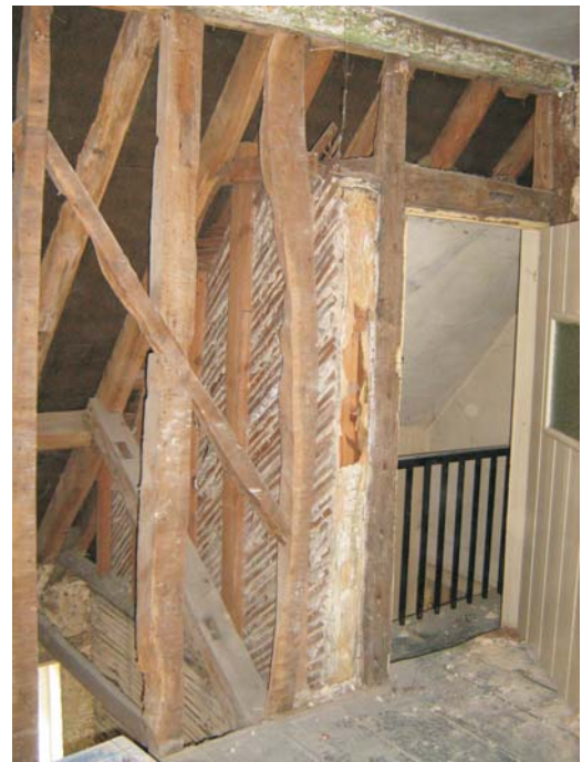
Plate 57: The south wall of bedroom 2 with raking strut to purlin of the outshot roof construction
