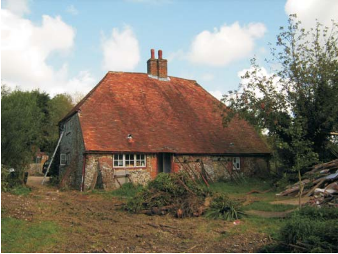
Plate 17: The external south elevation of the house shows 19th century brick quoins to the west window
