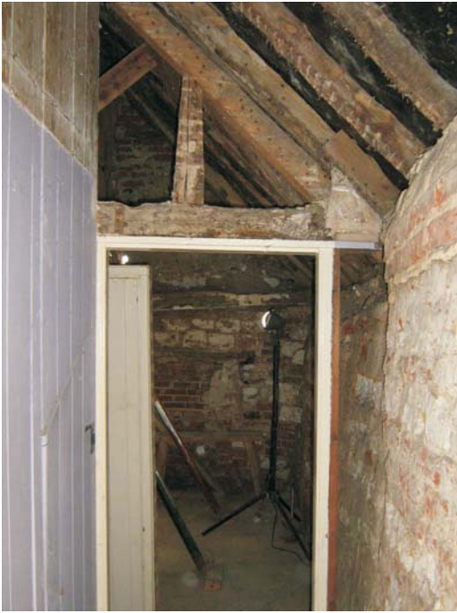
Plate 13: The south wall of the building with continuous chalk and brick construction - viewed through the doorway to the former bathroom
