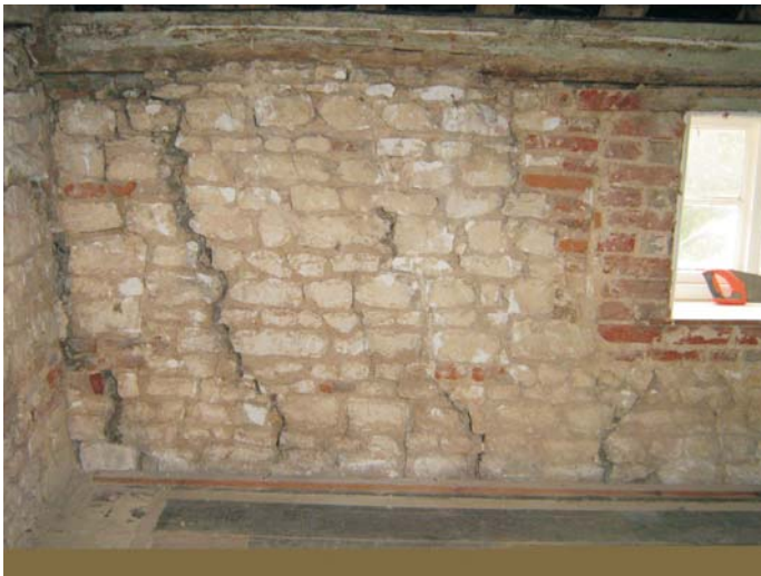
Plate 27: The west end of the north wall shows the substantial cracking of the chalk block masonry
