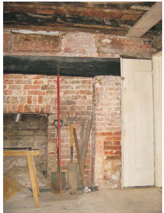
Plate 20: The south side of the inglenook with inserted cupboard under additional lintel
