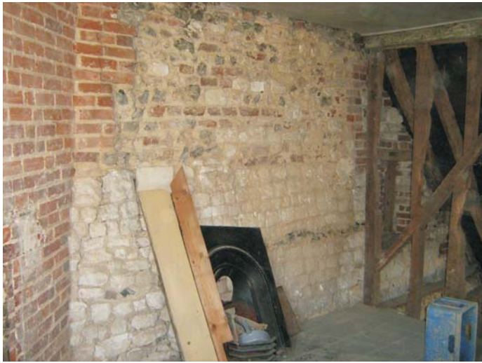
Plate 68: The contrast between the later brickwork and the earlier chalk block construction of the chimney breast and the east wall of bedroom 2
