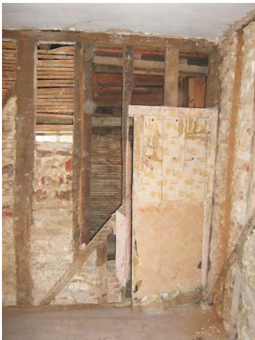
Plate 44: The south wall of the sitting room with inserted doorway overlain by successive layers of mid to late 20th century wallpaper when the door was no longer in use
