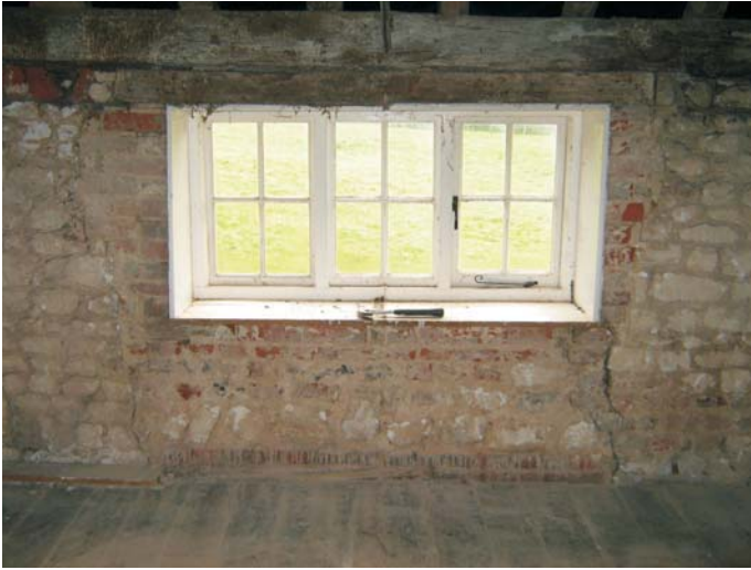
Plate 29: The east wall of bedroom 2 shows window inserted into the formerly un-breached fabric - shows a 19th century casement
