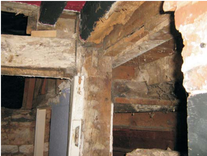
Plate 9: The timber beam across the front of the living room fireplace, jointed into the post of the original frame
