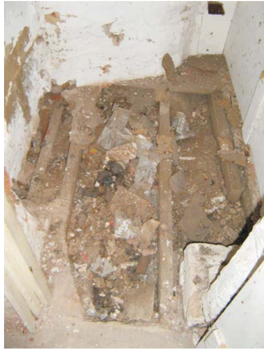
Plate 22: The floor of the cupboard after the removal of the covering plywood boards
