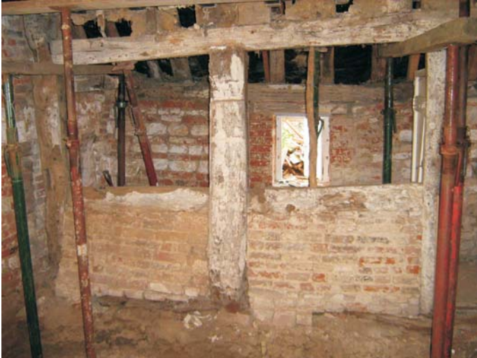
Plate 5: The lower panels of the south wall, fully stripped to reveal the later brick in-fill
