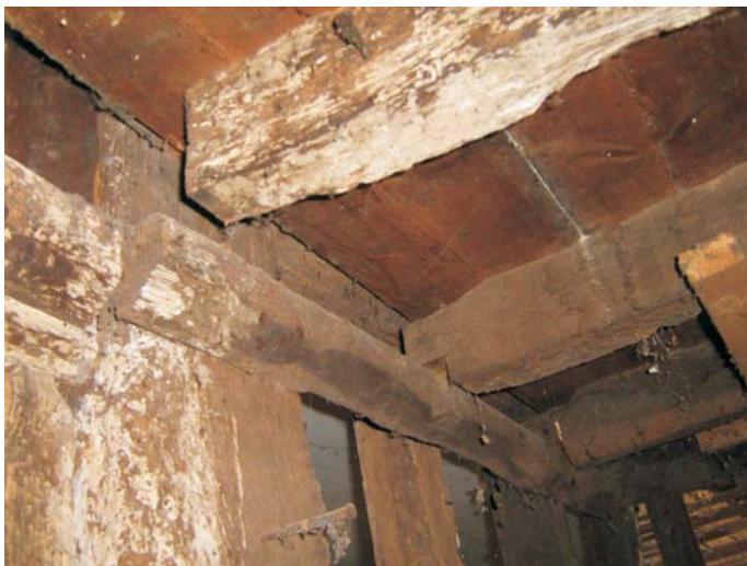
Plate 54: Added timber member attached to south side of the timber partition wall between sitting room and bathroom, to support the stair construction
