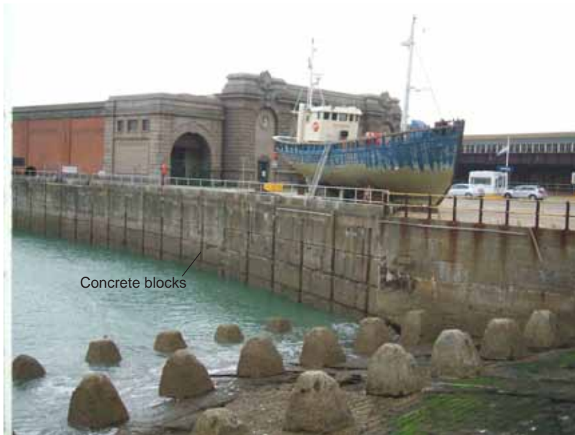
Fig. 8.1 Concrete blocks in wall of Admiralty Pier, Dover harbour (Photo: R. Cole)
