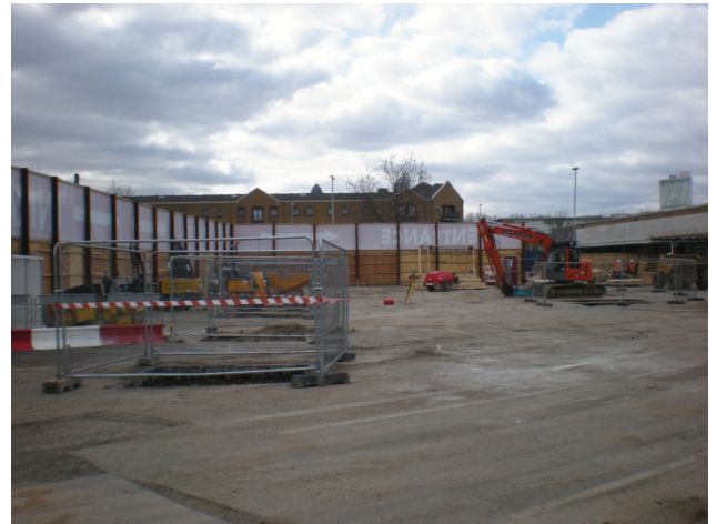
DP 2. Central part of the site with trenches for foundation pads. View SW.
