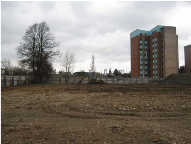
DP 1. Oldchurch Hospital site, Romford. NW part of the site. View NW.
