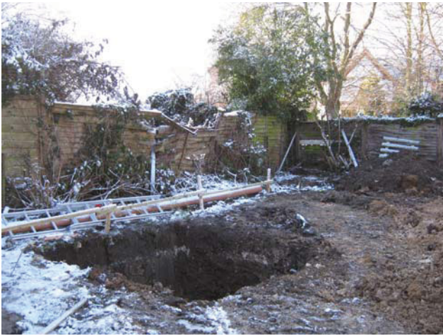
DP 9. Trench for a new soakway, S part of the site. View SW.
