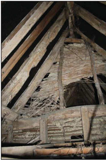
93 View of the roof space above Room FF04 showing the bay division (south bay, north range), taken from the south
