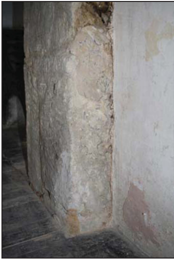
55 Detail of east fire-place jamb in Room FF01 showing original decorative paint scheme, taken from the south
