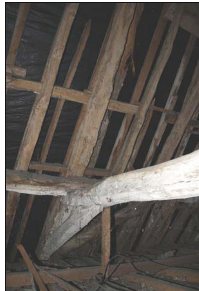
88 View in the roof space above Room FF01 (north bay, mid-bay division), taken from the north-west
