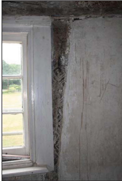
61 Detail of east wall in Room FF01 showing original decorative paint scheme, taken from the west
