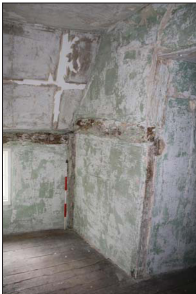
63 East side of Room FF03 in the north range, taken from the west
