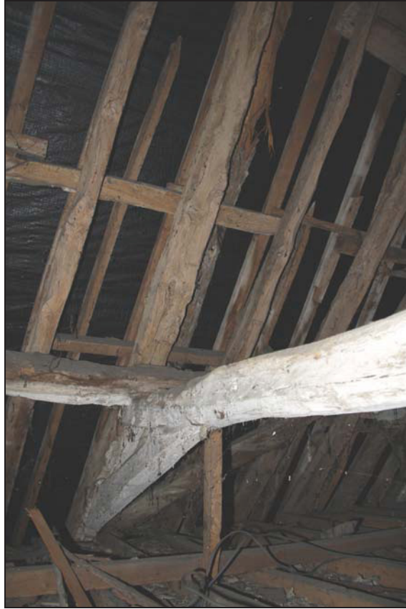
Plate 11 View in the roof space above Room FF01 (north bay, mid-bay division), taken from the north-west (88)
