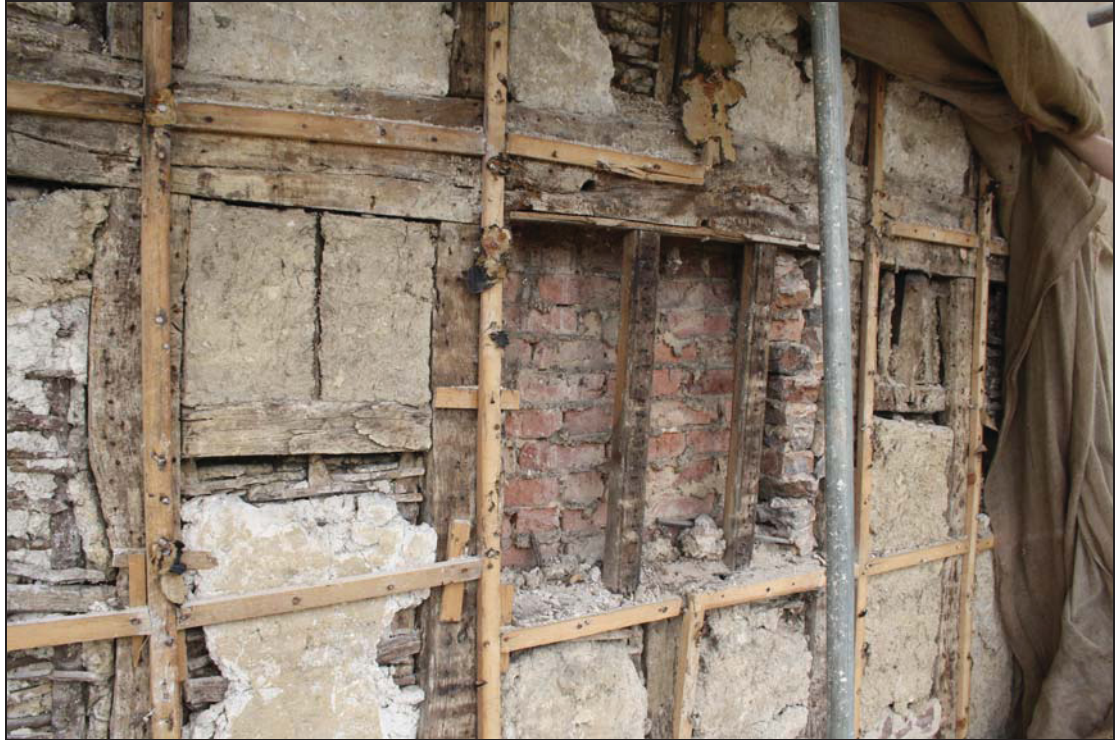
Plate 3 Blocked original tri-partite first-floor window on the south wall (south range), taken from the south-west (83)
