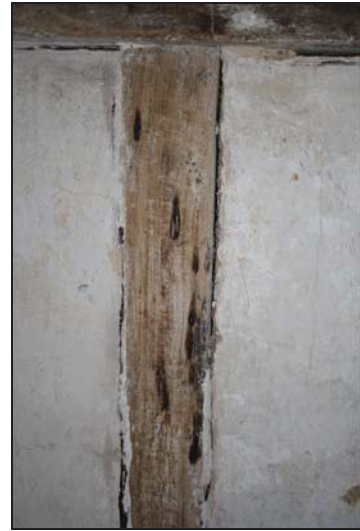
56 Stud on north wall of Room FF01 showing taper marks, taken from the south
