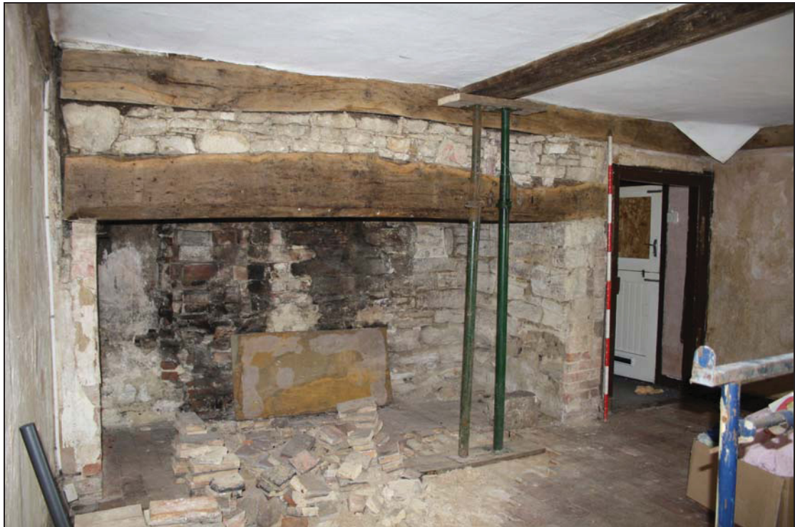
Plate 4 Inglenook fireplace on the north side of Room GF01, taken from the east (23)
