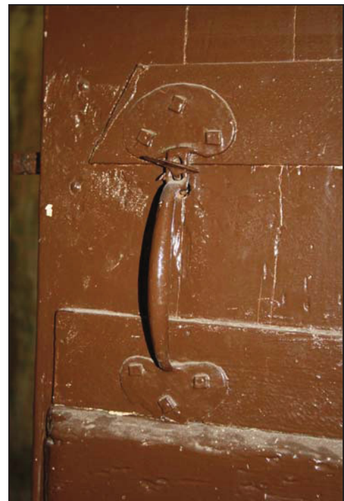
30 Upright handle on the west door, north wall of Room GF04, taken from the south
