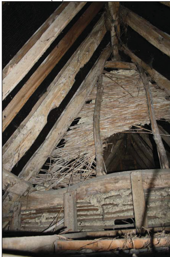
Plate 12 View of the roof space above Room FF04 showing the bay division (south bay, north range), taken from the south (39)
