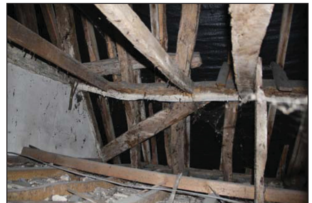
90 View of the roof space above Room FF01 (north bay, east side of the south range), taken from the west
