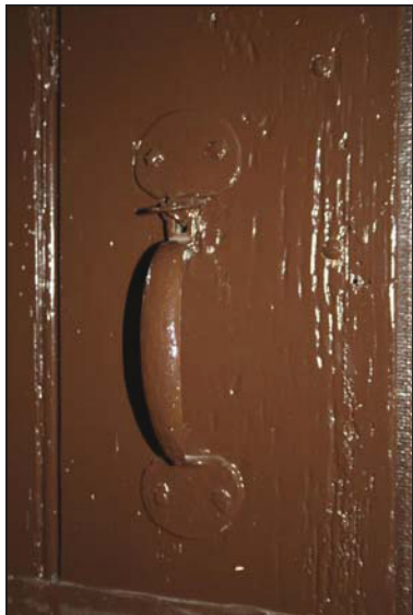
31 Upright handle on the east door, north wall of Room GF04, taken from the west
