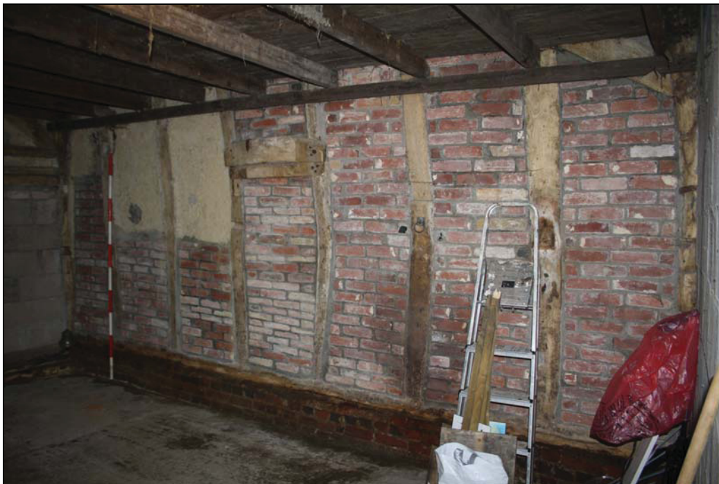
Plate 7 Interior of the east wall of the barn, taken from the south-west (DP 11)
