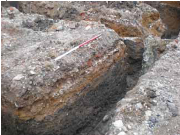
DP 5. Southern part of Building Plot A, western foundation trench (southern part) (Sample Section 2). View SE.
