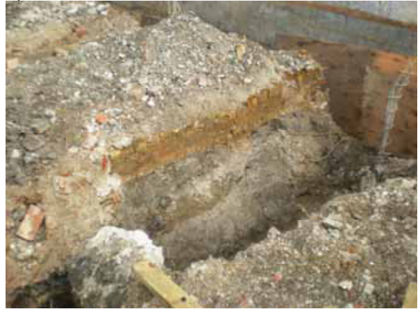
DP 4. Southern part of Building Plot A, southern foundation trench. Wall M1028. View NE.
