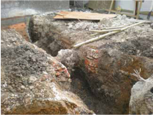
DP 3. Southern part of Building Plot A, southern foundation trench (Sample Section 1). View SE.
