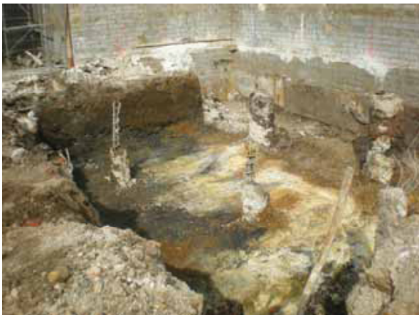
DP 9. Northern part of Building Plot A (area of 'strip, map & record'). View NNE.
