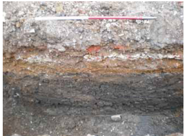
DP 6. Southern part of Building Plot A, western foundation trench (southern part) (Sample Section 2). View ENE.
