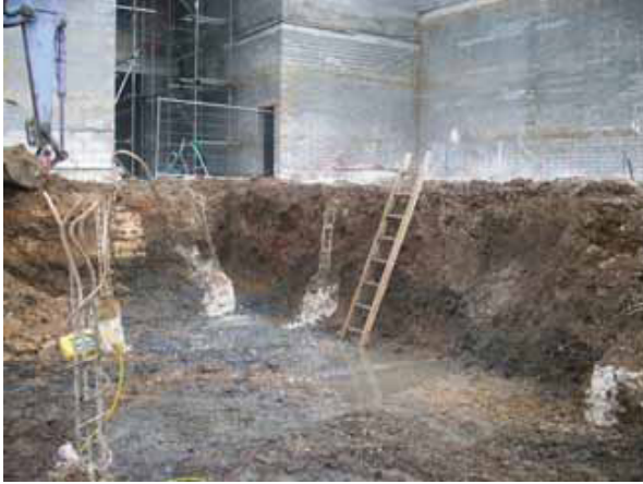
DP 13. Building Plot B (area of 'strip, map and record'). View N from south end.
