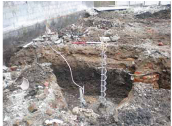
DP 2. Southern part of Building Plot A, northern foundation trench (Sample Section 3). View SSE.
