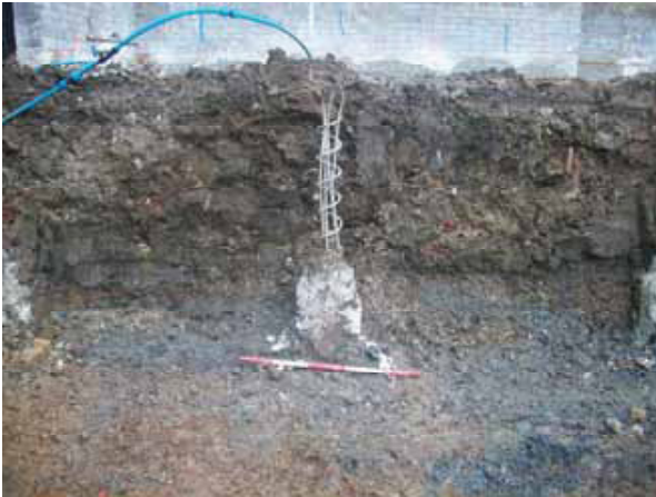
DP 15. Building Plot B (area of 'strip, map and record'), south-west-facing section (Sample Section 6), southern part. View ENE.
