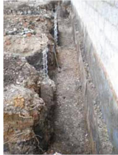
DP 8. Southern part of Building Plot A, eastern foundation trench. View NNW.
