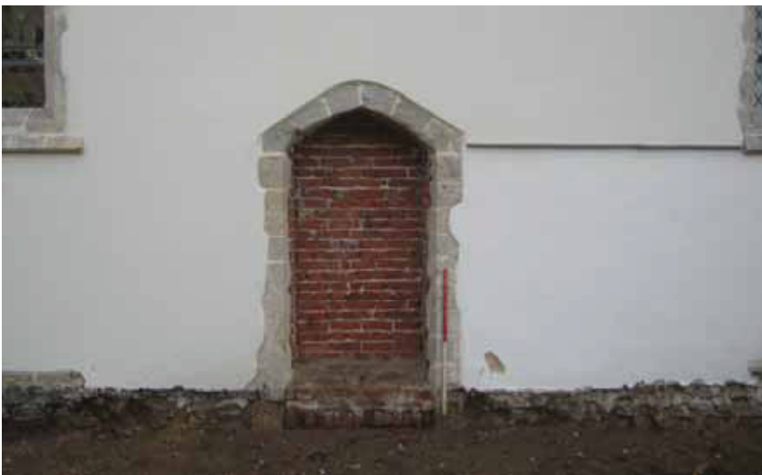
9 North elevation of chancel, vestry wall nubs M1008 and M1009 visible beneath render. Looking south.
