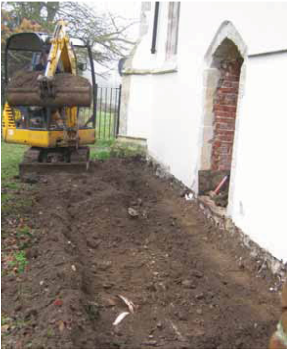
7 General view of topsoil excavation beside north wall of chancel. Looking east.
