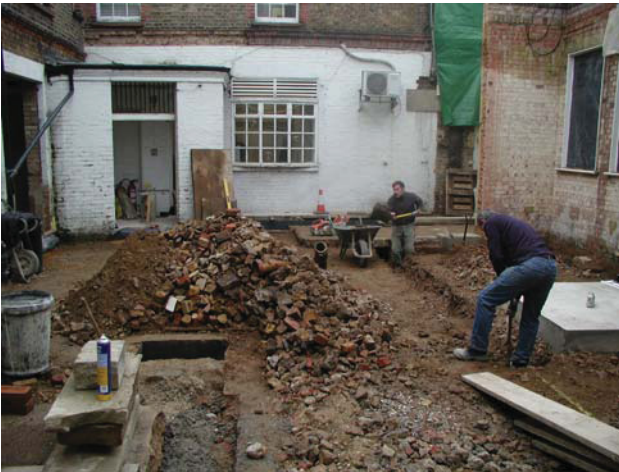
DP 1. The Old Police Station, Hertford. SW yard within the building. View E.
