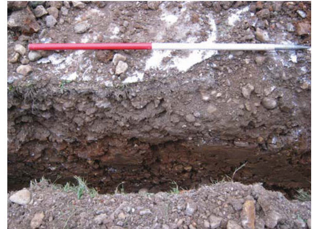
DP 4. Water main trench to the north of the house. Sample section. View W.
