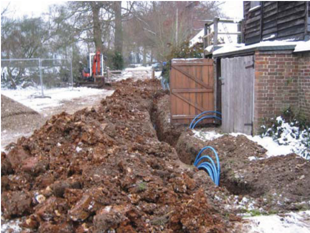
DP 3. Water main trench to the north of the house. View NNE.
