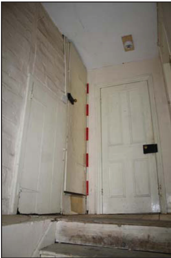
63 First floor landing (FF07) with doors leading to a small cupboard, the attic stair and FF06, taken from the north-east
