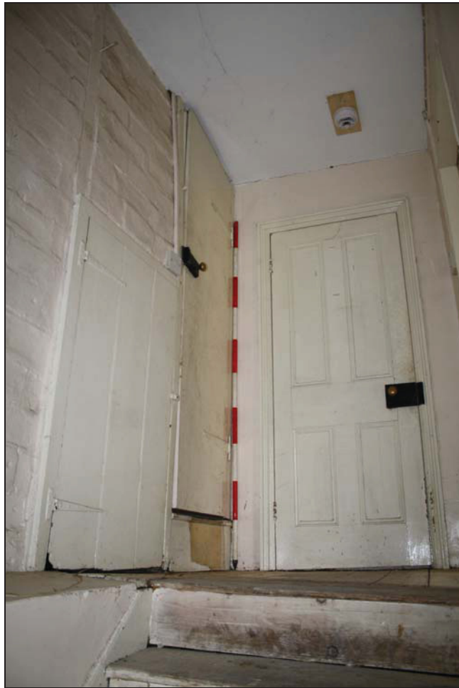
Plate 19 First floor landing (FF07) with doors leading to a small cupboard, the attic stair and FF06, taken from the north-east (DP 63)
