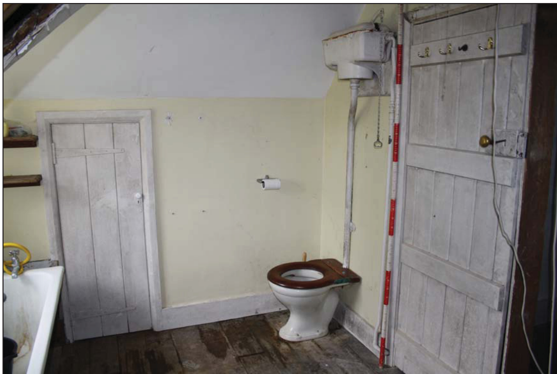
Plate 23 Bathroom retaining early 20th century fixtures and fittings, SF09, taken from the north-west (DP 145)
