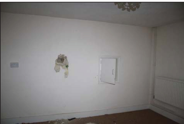
65 East wall of Room GF02 (Building 2) showing intervention to exposed historic fabric, taken from the north-west
