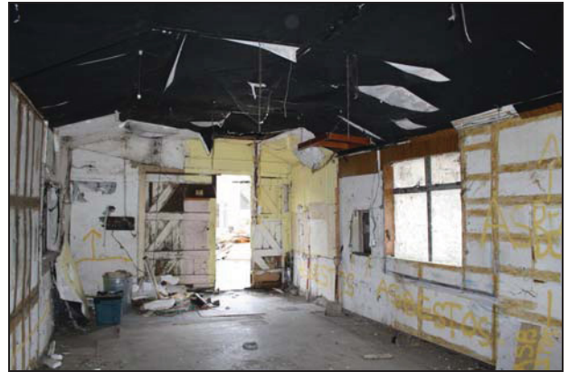
80 Interior of Building 3 after soft-stripping of internal elements, taken from the north
