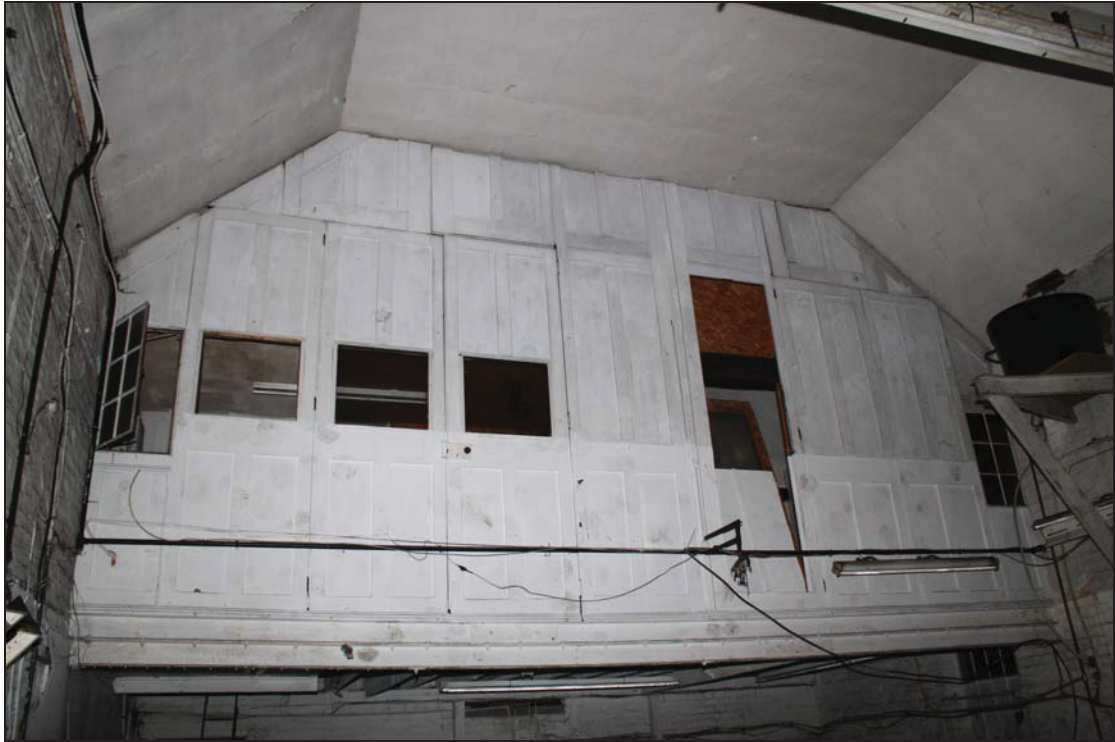
5 Panelled partition enclosing the mezzanine level in Building 1, taken from the west (38)
