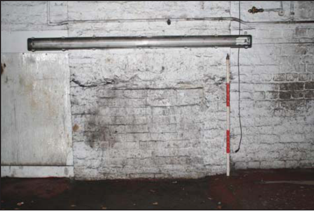
43 Detail of the western blocked fireplace on the east wall of the main range (Building 1), taken from the north
