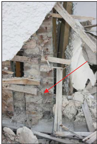
89 Assembly mark (indicated) on a bay post of the west wall of Building 2 exposed during demolition, taken from the west
