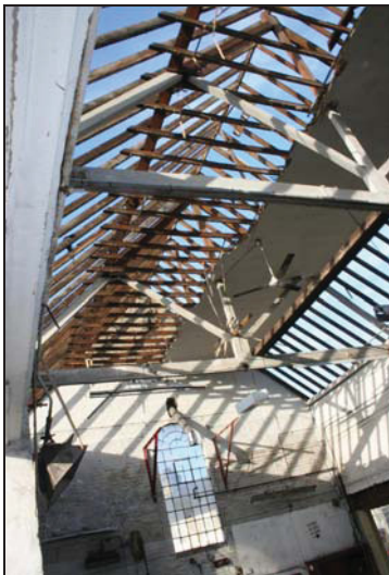
95 View of the west end of Building 1 (main range) after removal of the ceiling and exposure of the roof trusses, taken from the east
