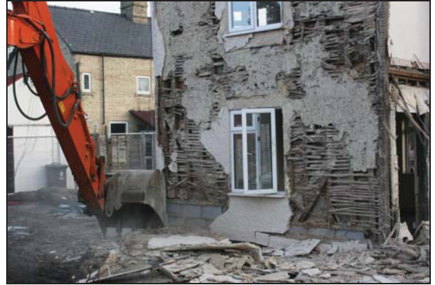
92 External west wall of Room GF01 (Building 2) showing primary-braced studwork and surviving lath and plaster, taken from the west
