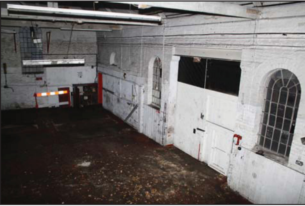
55 View of the main range of Building 1 viewed from the mezzanine level, taken from the east
