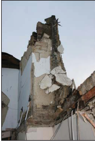
87 View of chimney stack at the south end of Building 2, truncated at eaves level, taken from the west
