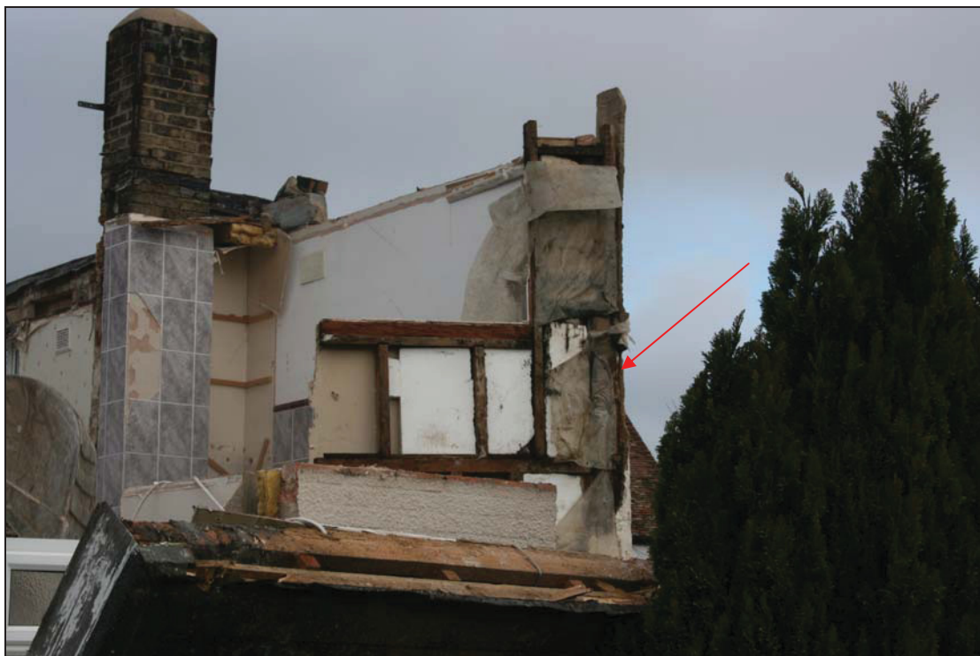
9 South end of the rear range (Building 2) during demolition showing surviving timber elements (indicated) with later timber repair, taken from the south-west (74)
