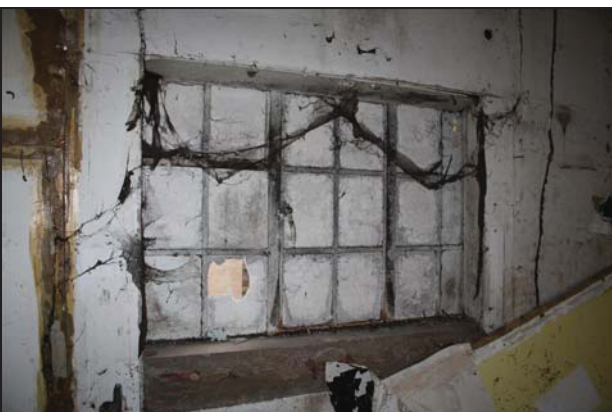
83 Formerly hidden window on the east wall of Building 3, taken from the west
