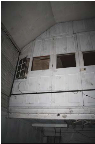
63 Detail of partition enclosing the mezzanine in Building 1, taken from the west
