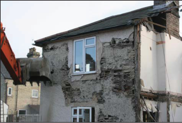
91 External west wall of Room GF01 (Building 2) showing primary-braced studwork and surviving lath and plaster, taken from the west
