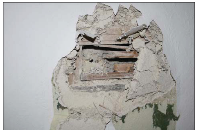
66 Detail of lath and plaster on the east wall of Room GF02 (Building 2), taken from the west
