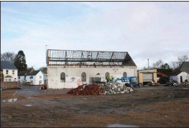
93 View of Building 1 after the removal of the roof covering and rear range, taken from the south
