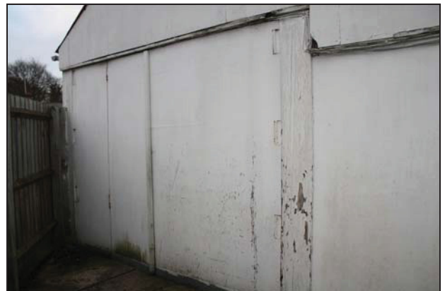
72 North wall of Building 3 showing double doors (no longer in use), taken from the south-east
