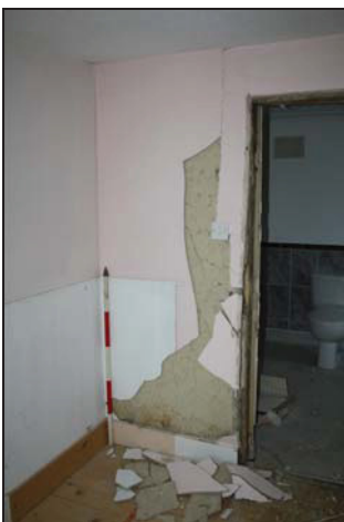
77 East wall of Room FF03 (Building 2) showing exposed studwork covered with lath and plaster, taken from the south-west
