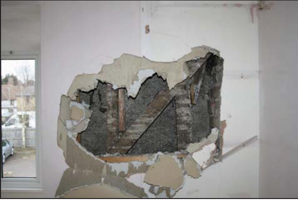
85 North wall of Room FF01 (Building 2) showing primary-braced studwork, taken from the south
