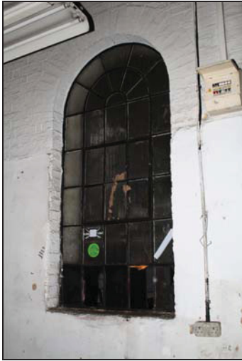
45 Window on the south wall of Building 1 from within the rear range, taken from the south-east
