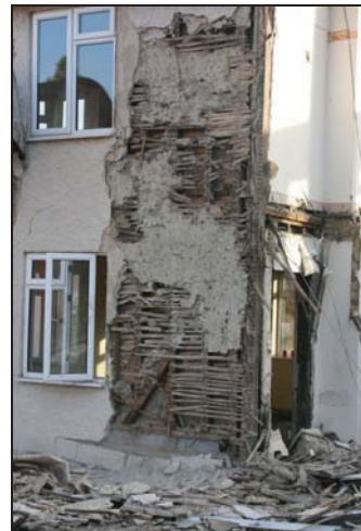
90 External west wall of Room GF01 (Building 2) showing primary-braced studwork and surviving lath and plaster, taken from the west
