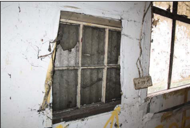
81 Formerly hidden window on the west wall of Building 3, taken from the south-east
