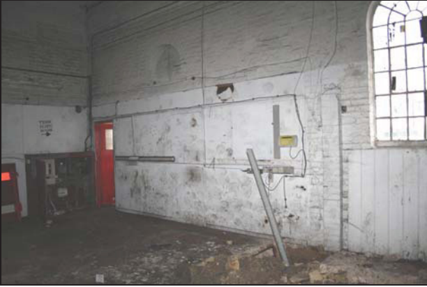
61 West end of the north wall of the main range (Building 1), taken from the east
