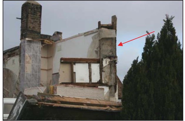
74 South end of the rear range (Building 2) during demolition showing surviving timber elements (indicated) with later timber repair, taken from the south-west
