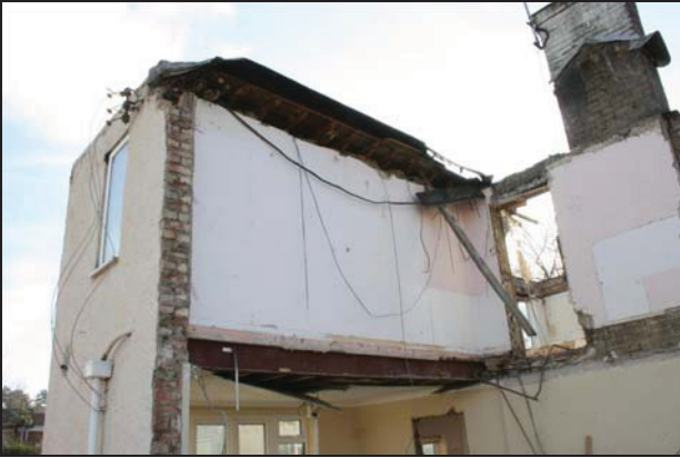
73 North end of the rear range (Building 2) during demolition showing Fletton brick construction, taken from the west
