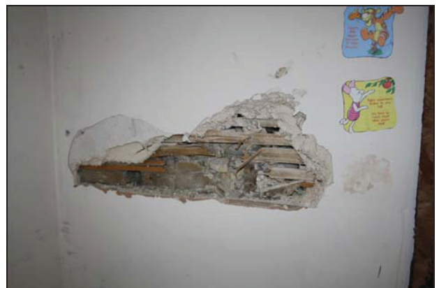
84 West wall of Room GF04 (Building 2) to the south showing exposed studwork covered with lath and plaster, taken from the north-east
