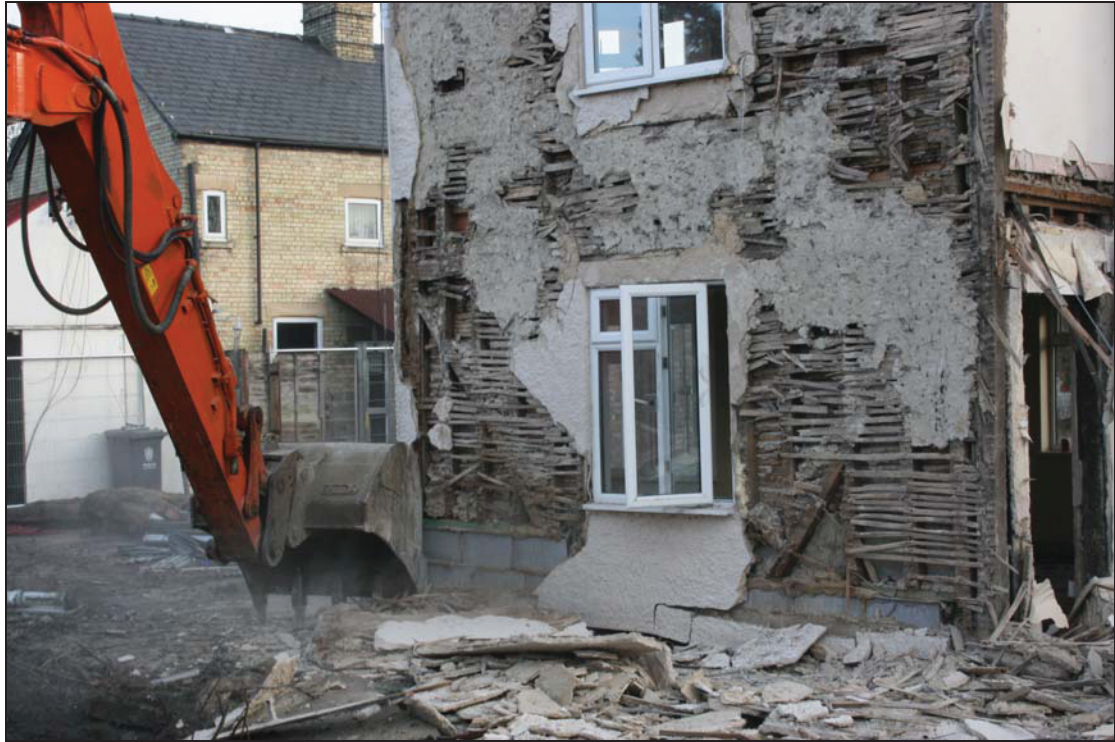
7 External west wall of Room GF01 (Building 2) showing primary-braced studwork and surviving lath and plaster, taken from the west (92)
