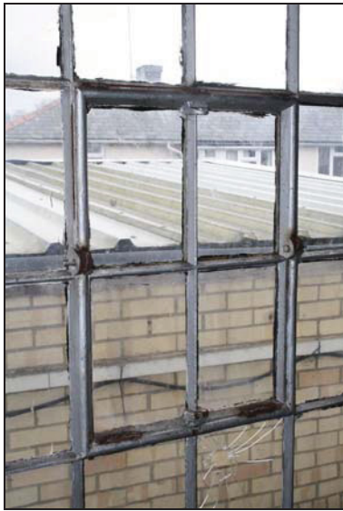
57 An example of a pivoting casement utilising the four central panes of the east window of Building 1, taken from the north-west
