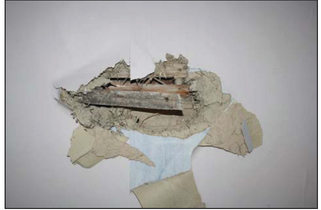
68 Detail of lath and plaster on the south wall of Room FF03 (Building 2), taken from the north
