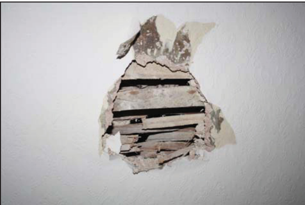
75 Detail of lath and plaster on the south wall of Room GF02 (Building 2), taken from the north
