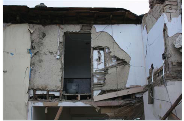
86 East wall of Room FF03 (Building 2) during demolition showing original studwork and lath and plasterwork, taken from the west
