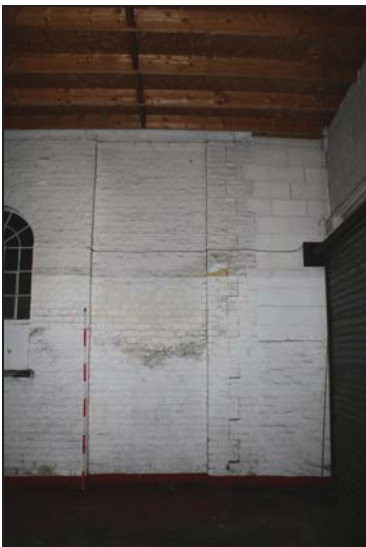
47 West end of the south wall of Building 1 from within the rear range, taken from the south
