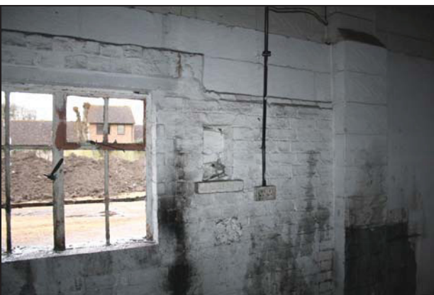
59 Detail of blocked aperture on the north wall of the rear range (Building 1), taken from the north-east
