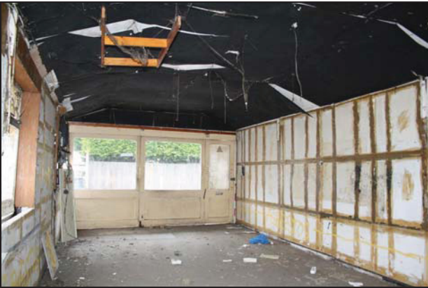
79 Interior of Building 3 after soft-stripping of internal elements, taken from the south
