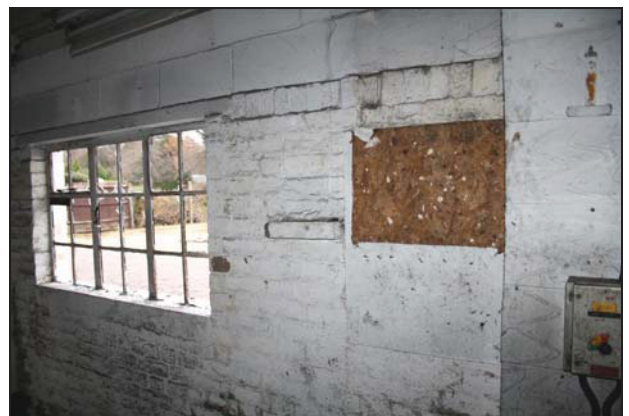
60 Detail of second blocked aperture on the north wall of the rear range (Building 1), taken from the north-west
