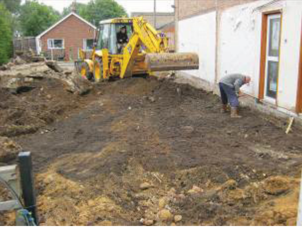
1 General view of the site during clearance of demolished footings and site grading. Looking north east.
