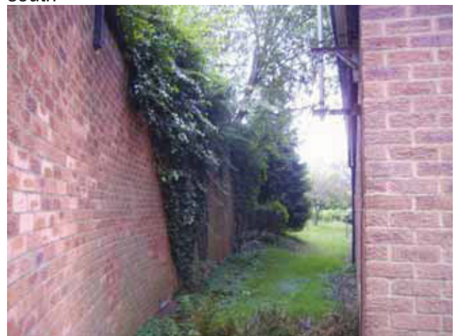
DP 12 Eastern boundary of the site comprising the eastern frontage of St Andrew's House, an extensive brick retaining wall and a small area of grass between
