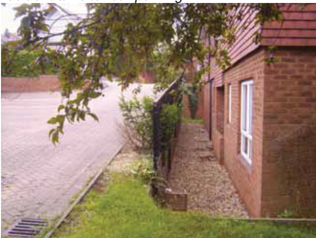
DP 9 North-western corner of St Andrew's House with an area of shingle at its base, confirming it had been cut into the natural ground level in comparison to the parking area
