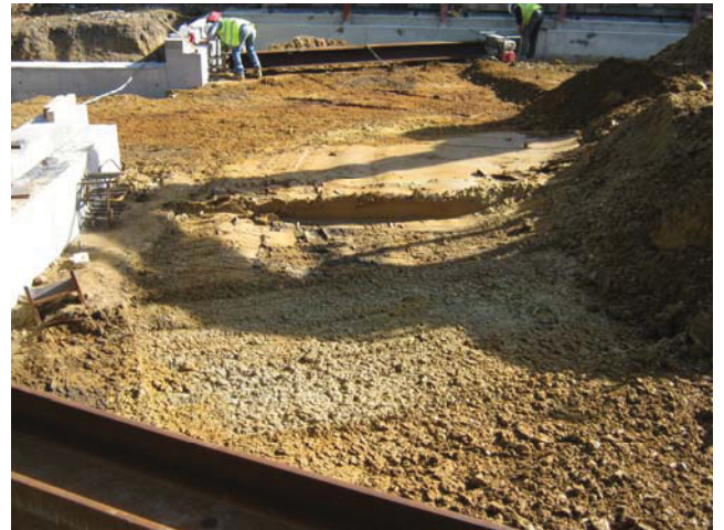
DP 10. W part of the site. Area of ground reduction. View NNE.
