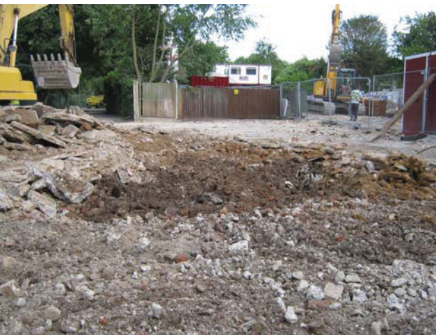
DP 5. The site during removal of existing paving and foundations. View E.
