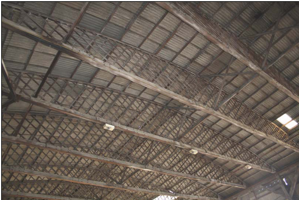
Plate 10 Belfast roof trusses, interior, south-eastern unit, Building 6, taken from the south-west (DP 199)
