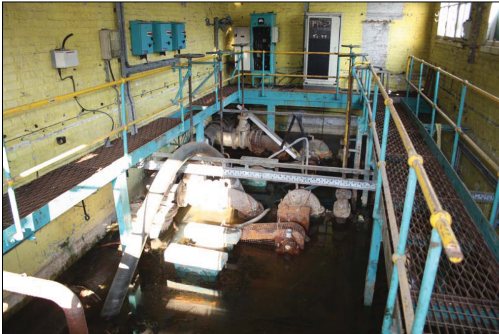
Plate 32 Lower tank, the pump house, Building 17, taken from the south-east (DP 58)
