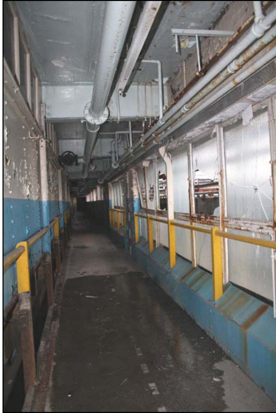
Plate 21 Corridor and tanks, first floor mezzanine, south side of Building 10, taken from the west (DP 119)
