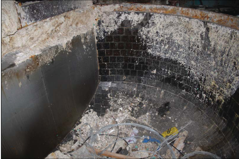
Plate 7 Interior of hydro-pulper lined with ceramic tiles, first floor, eastern end of Building 4, taken from the north-west (DP 238)
