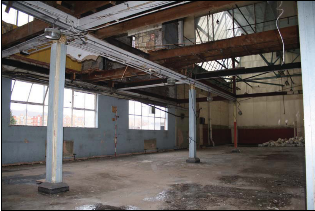
Plate 19 Interior of enclosed northern side of Building 10, taken from the south-west (DP 116)
