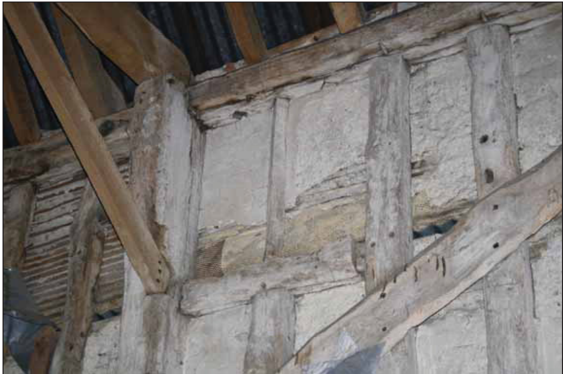
Plate 7 Original upper window on the east side of Bay 5 (Building 1) with original diamond profile mullion, taken from the south-west (DP 51)
