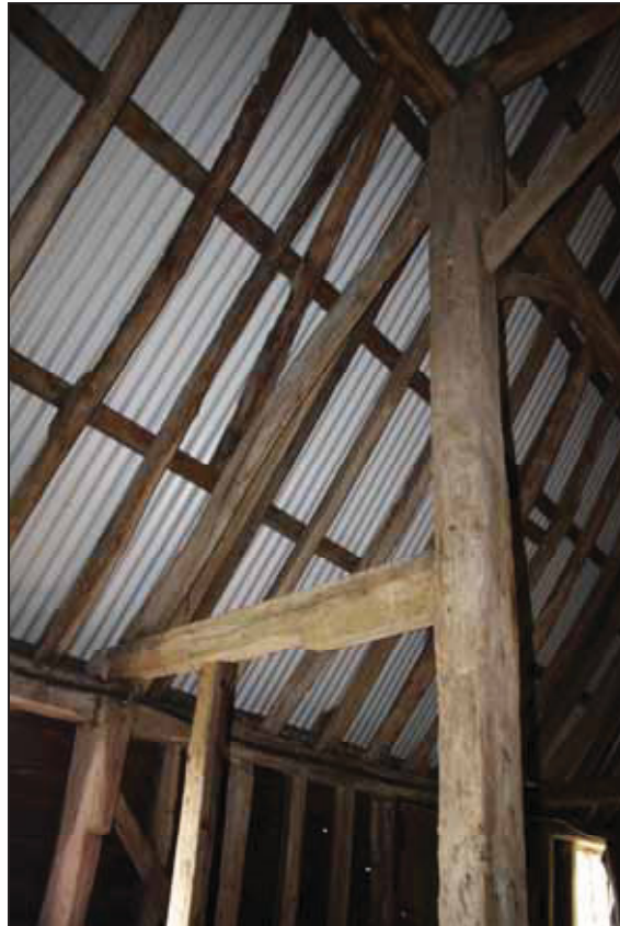
Plate 9 West end of Truss 7 (Building 1) within the aisle, taken from the south-east (DP 62)
