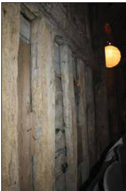
DP 47 Studwork on the east side of Bay 2 showing wattle notches, taken from the north
