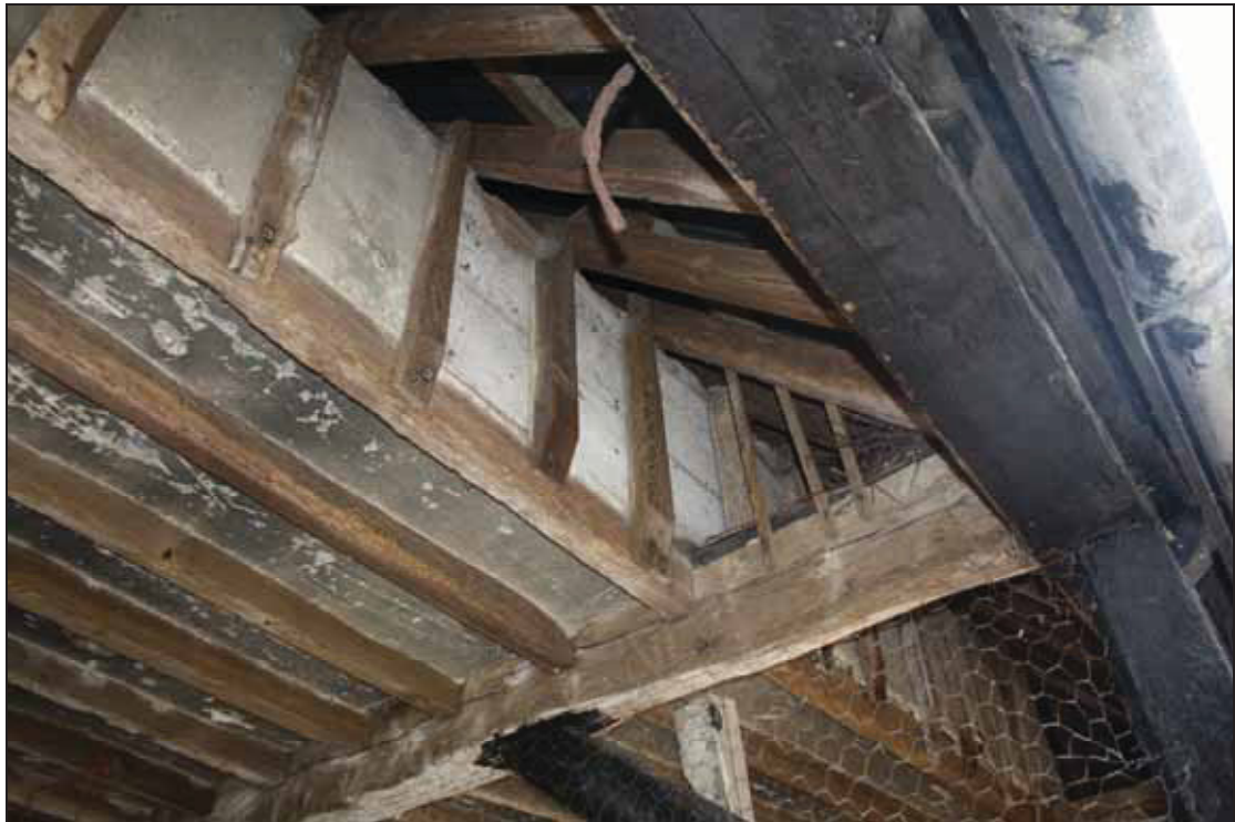
Plate 13 Studwork enclosing the eaves of the loft occupying the north two bays of Building 2, taken from the south-east (DP 75)
