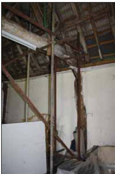
DP 29 West end of the truss between Bays 4 and 5 (Building 3), taken from the north-east
