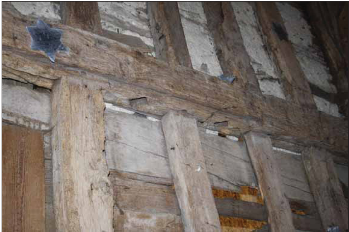
Plate 5 Position of original lower window on the east side of Bay 2 (Building 1), taken from the north-west (DP 46)
