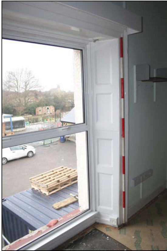
Plate 9 Splayed reveals and 18 th century type mouldings, west elevation, first floor, taken from the south-east (DP 23)
