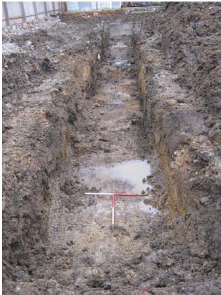
DP 7. Trench 3. View before collapsing. Looking south-east.
