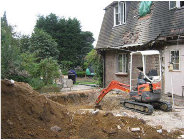
DP 1. The eastern side of the house with excavation area. Looking south-west.
