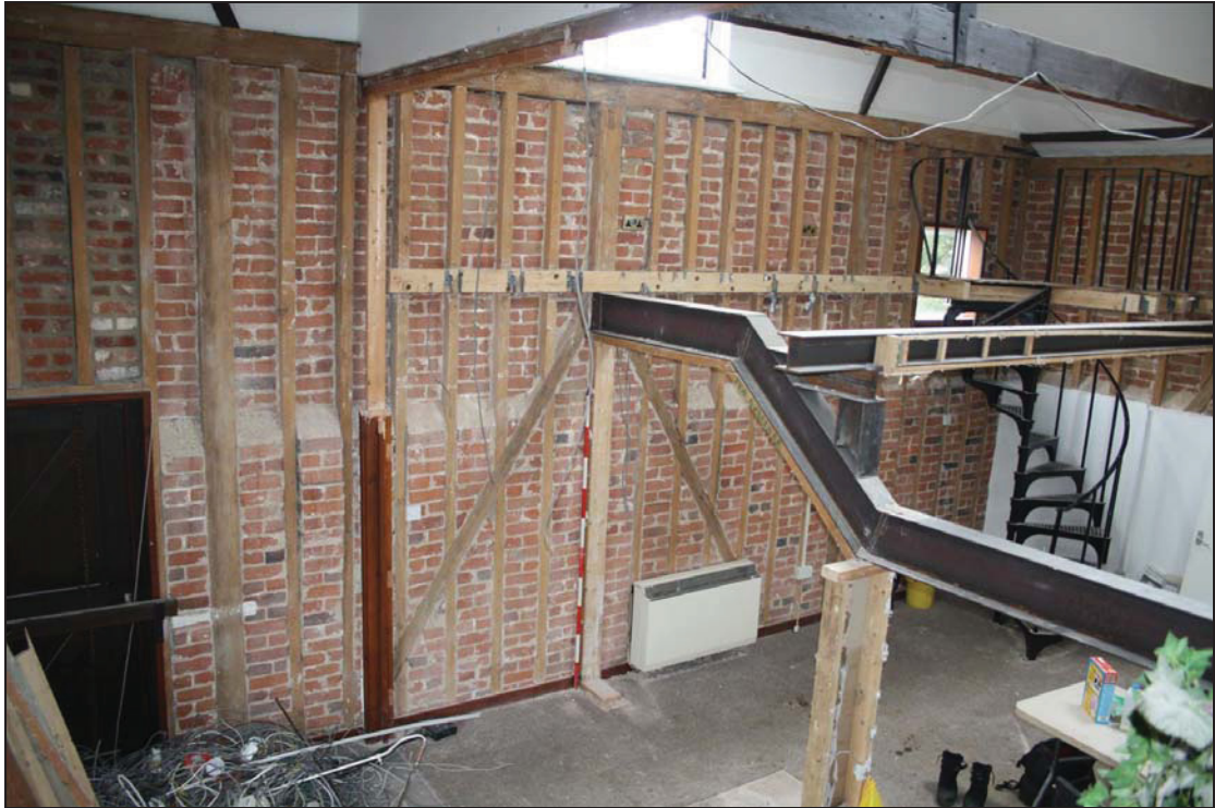
5 West wall of the steeping bays at upper level (Building 1), taken from the south-east (DP 89)
