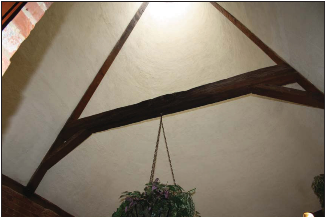
10 Truss of kiln cone above Room FF04 (south kiln in Building 1), taken from the south-west (DP 43)
