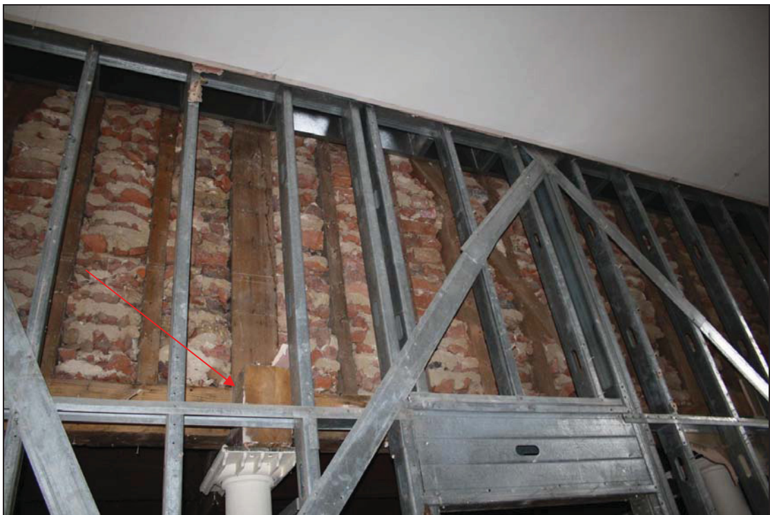
4 Detail of the junction between the steeping bays and malting floor showing truncated bridging joist (indicated) (Building 1), taken from the east (DP 81)
