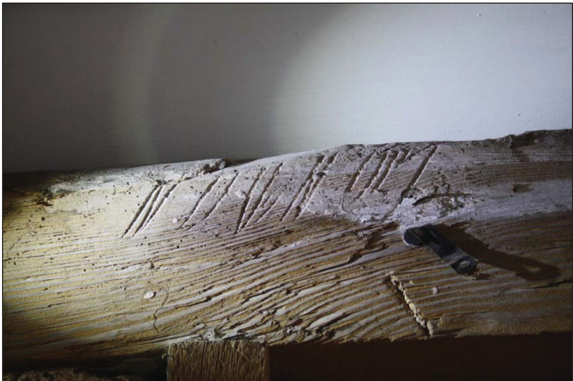
6 Baltic bracking mark on the south wall-plate of Room MF01 (Building 1), taken from the north (DP 32)
