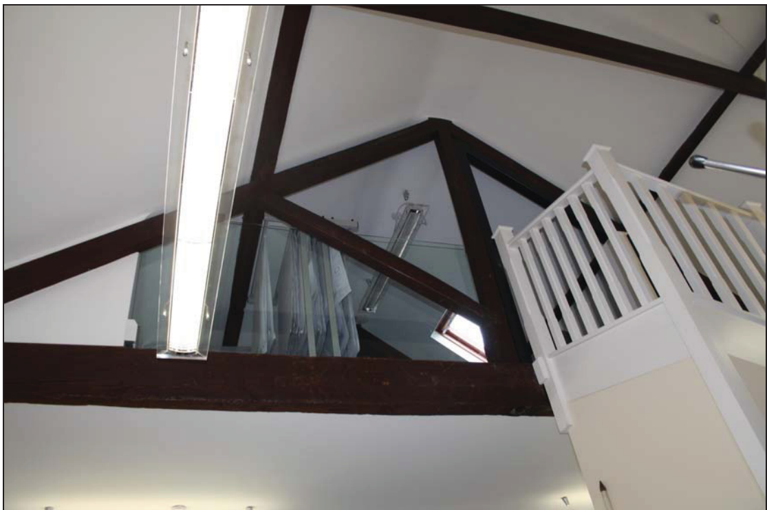
14 Roof structure over the north range of Building 2, taken from the south (DP 85)
