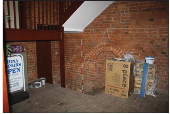
East side of Room GF07 (south kiln of Building 1), taken from the west
