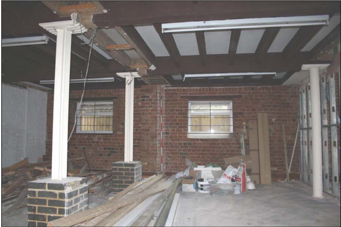
3 North side of the steeping bays at ground floor level (Building 1), taken from the south (DP 82)
