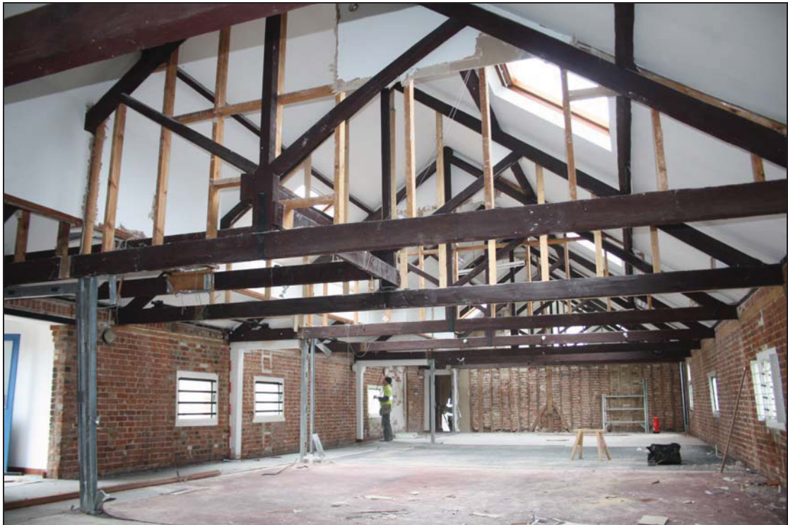
9 View of the upper former germination floor (Building 1), taken from the east (DP 104)
