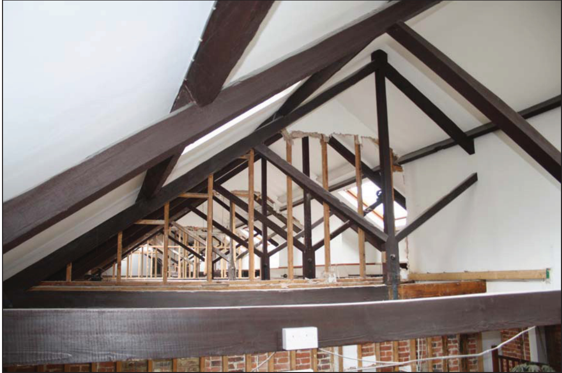
7 View of the roof structure over Building 1, taken from the west (DP 92)
