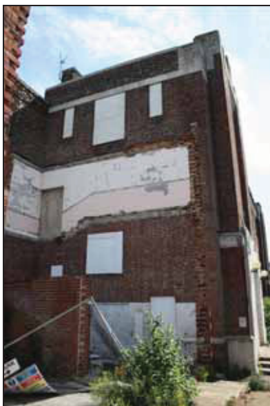
5 South-west corner of the Law Building showing area of removed building elements, taken from the west
