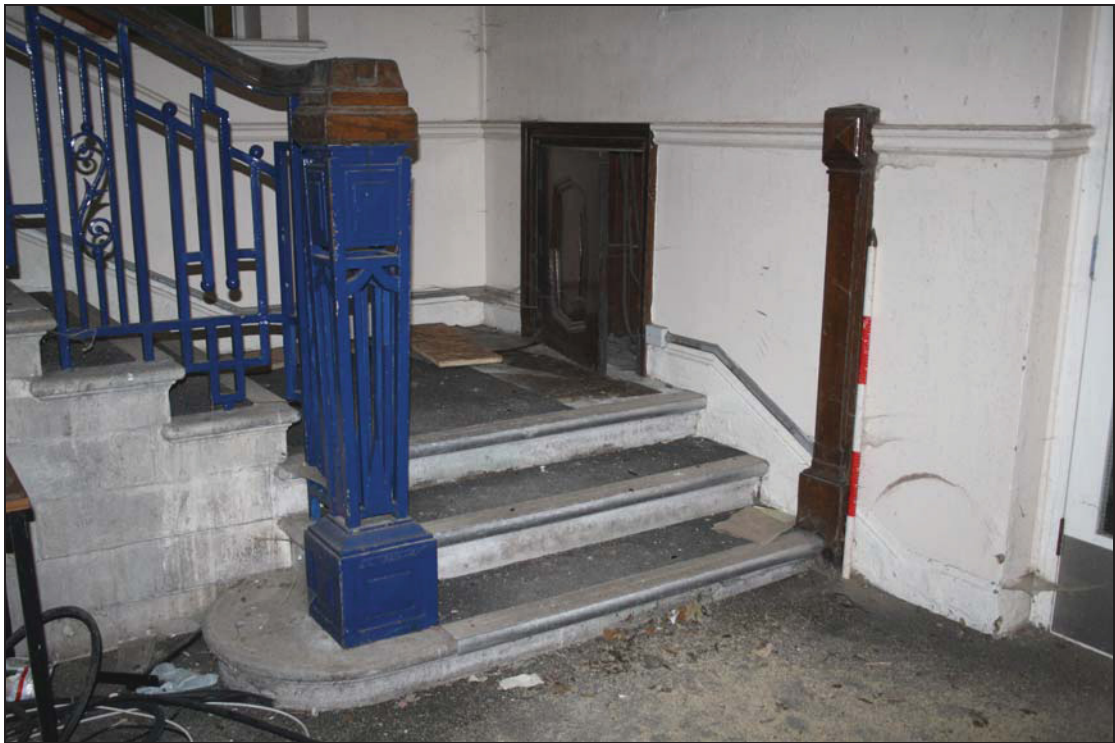
18 Apex of the early roof entombed within the existing structure showing formerly external plasterwork, taken from the west (85)
