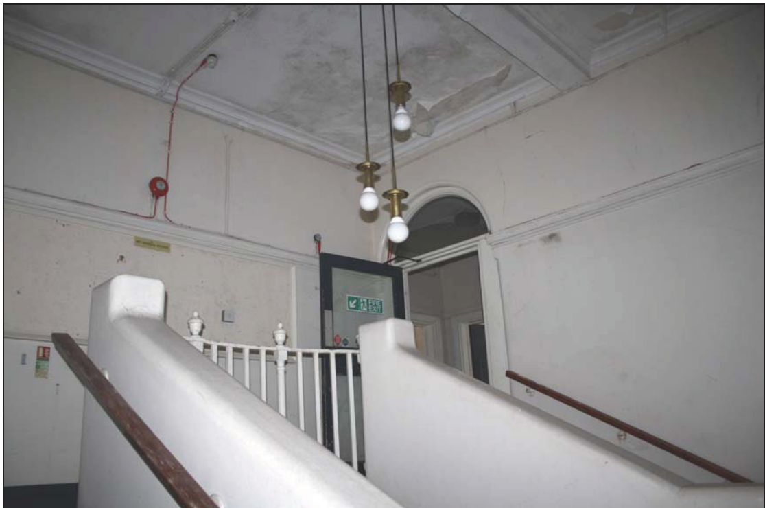
10 Stair landing FF01 from the half-pace landing (Frederick Chancellor Building), taken from the west (95)
