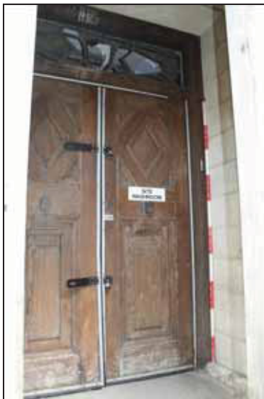
27 Doorway of the principal entrance to the Law Building, taken from the south-west
