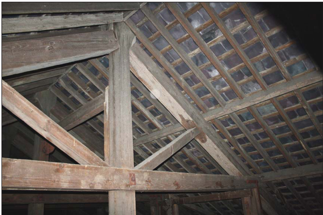
4 View of the roof structure over the Anne Knight Building, taken from the north-east (157)
