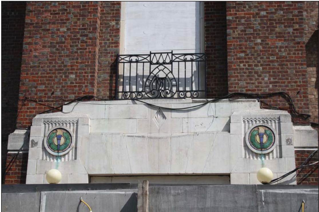
17 Detail of the principal entrance on the south side of the Law Building, taken from the south (15)
