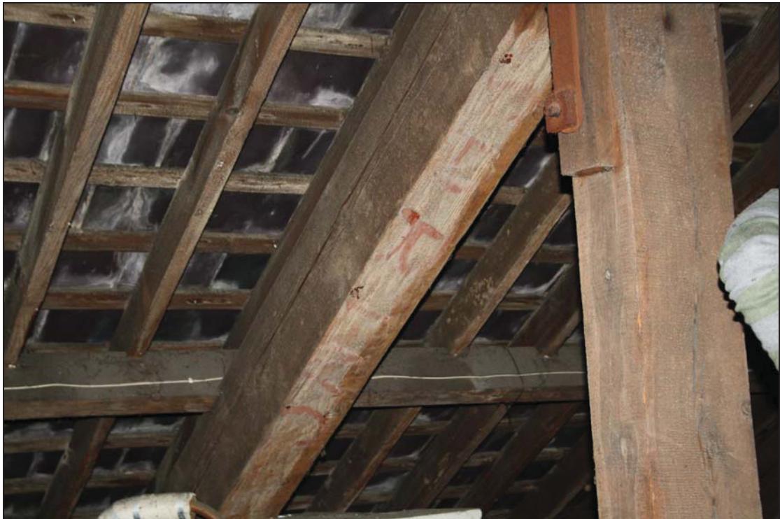
5 Painted batch mark on a principal rafter in the roof (Anne Knight Building), taken from the north-west (159)
