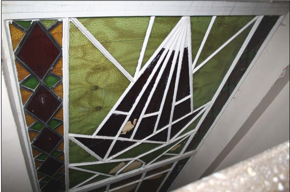
23 Stairlight on the second floor landing SF01 (Law Building), taken from the north (69)
