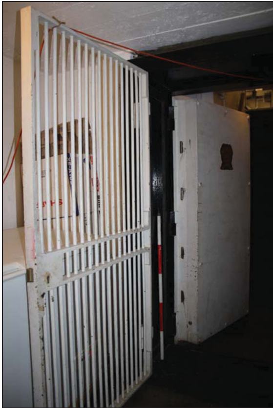
DP 29 Security doors to the basement underlying the north-east corner of the building, taken from the east
