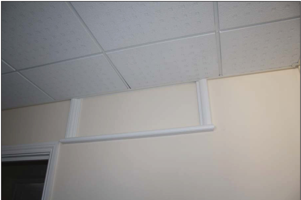
DP 25 Blocked aperture in the central corridor to Room FF04, may conceal earlier fabric, taken from the east
