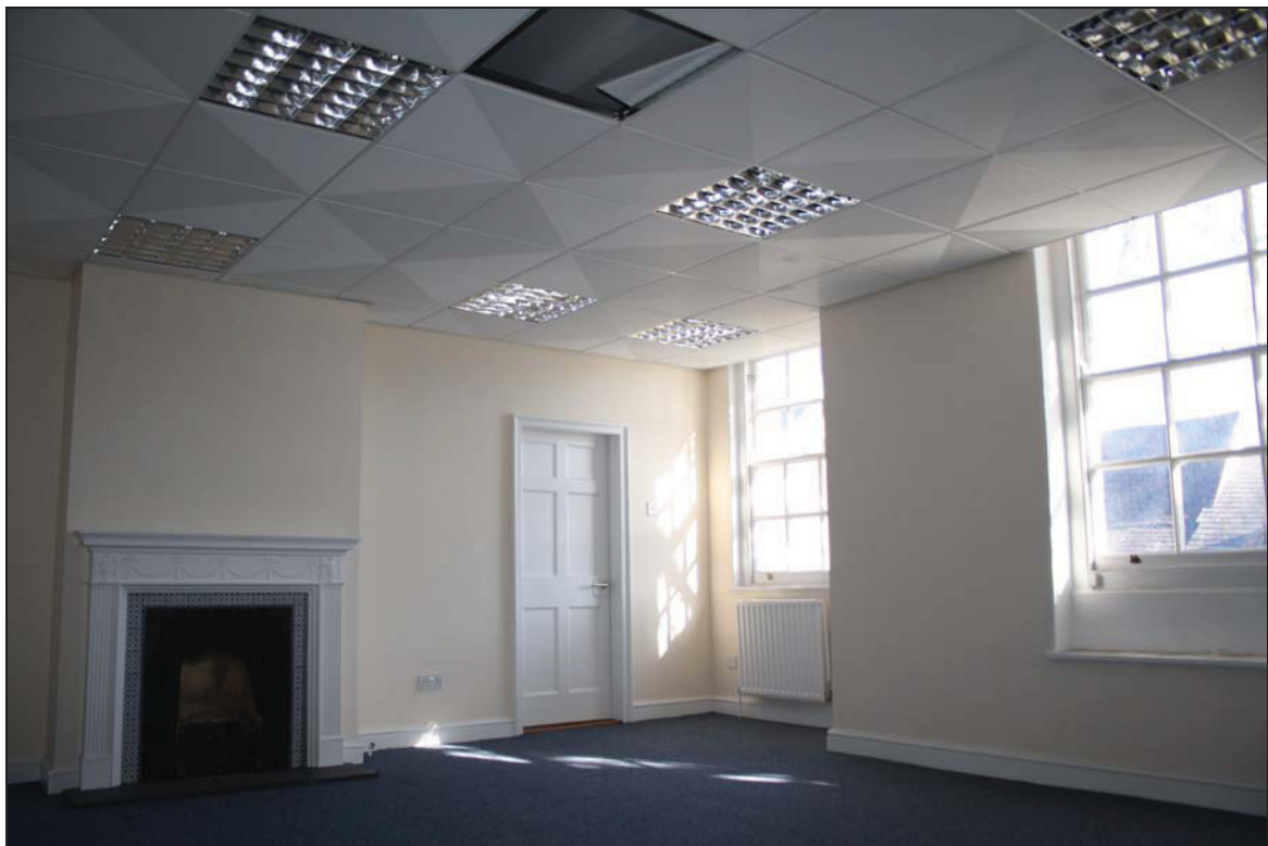
DP 23 View of Room FF03 with early 20 th century inset tiles but a modern replacement chimneypiece, early doorway to Room FF02 and windows with replacement sashes, taken from the south-west
