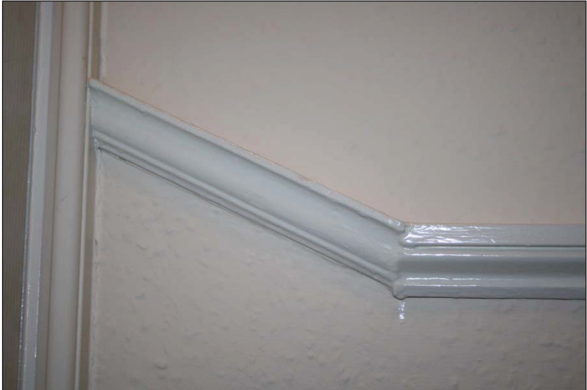
DP 32 Detail of the dado rail on the first floor landing (FF01) showing the original rail on the left with the later replacement on the right, taken from the west
