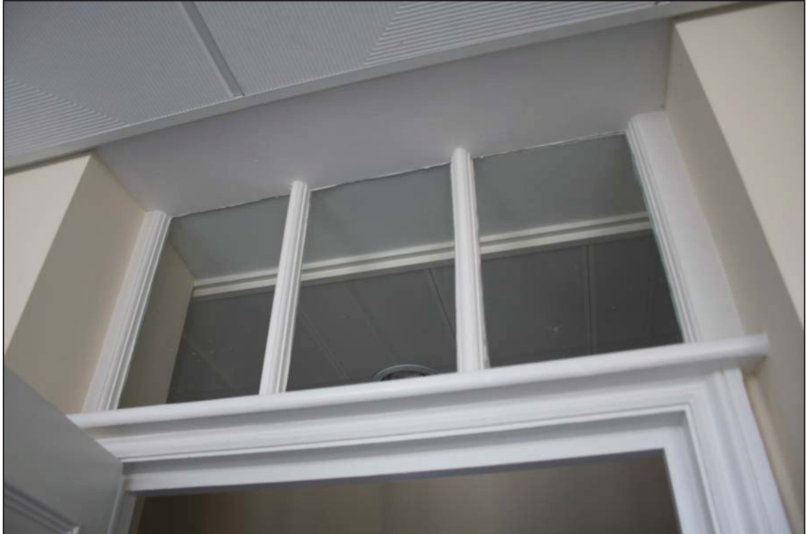
DP 24 Overlight in Room FF03 to the central corridor, possibly replaced but following an earlier form, taken from the east
