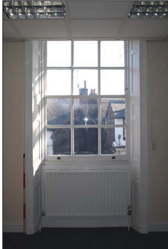
DP 16 Full height window embrasure with probable late 18 th or early 19 th century shutters and surround (sashes replaced) in FF02, taken from the west
