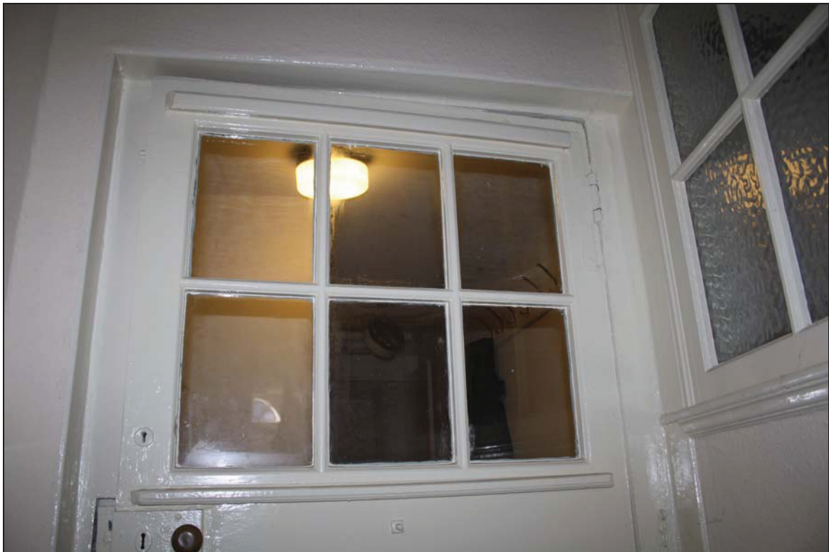
DP 12 Detail of the back door showing upper glazing and ledges for a removable shutter, taken from the east
