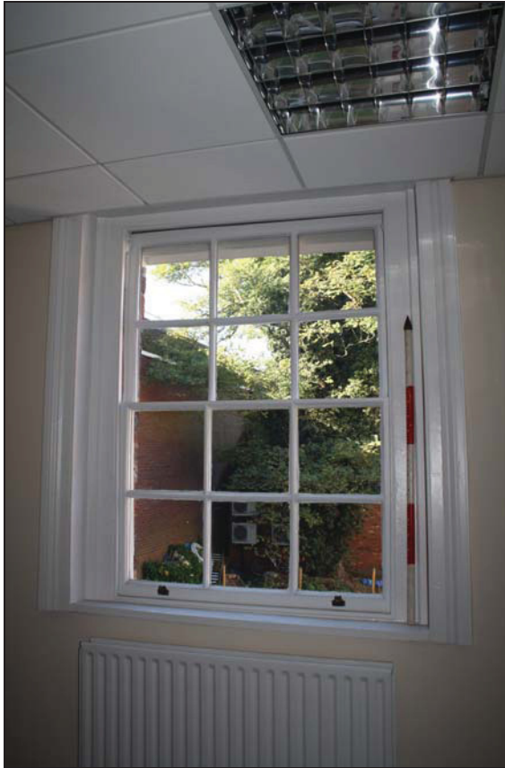
DP 26 Partially renewed window in Room FF05. 18 th century elements survive, for example the upper sash with characteristic 18 th century glazing bars, while the lower sash may be early but stripped of all paint history, taken from the north-east
