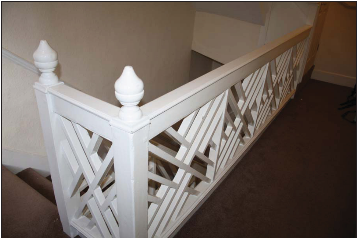
DP 33 View of the staircase at first floor level, this probably continues to second floor level now boxed in, taken from the south-west
