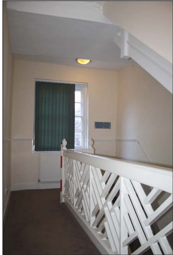
DP 14 First floor landing (FF01) showing stair balustrade, taken from the east
