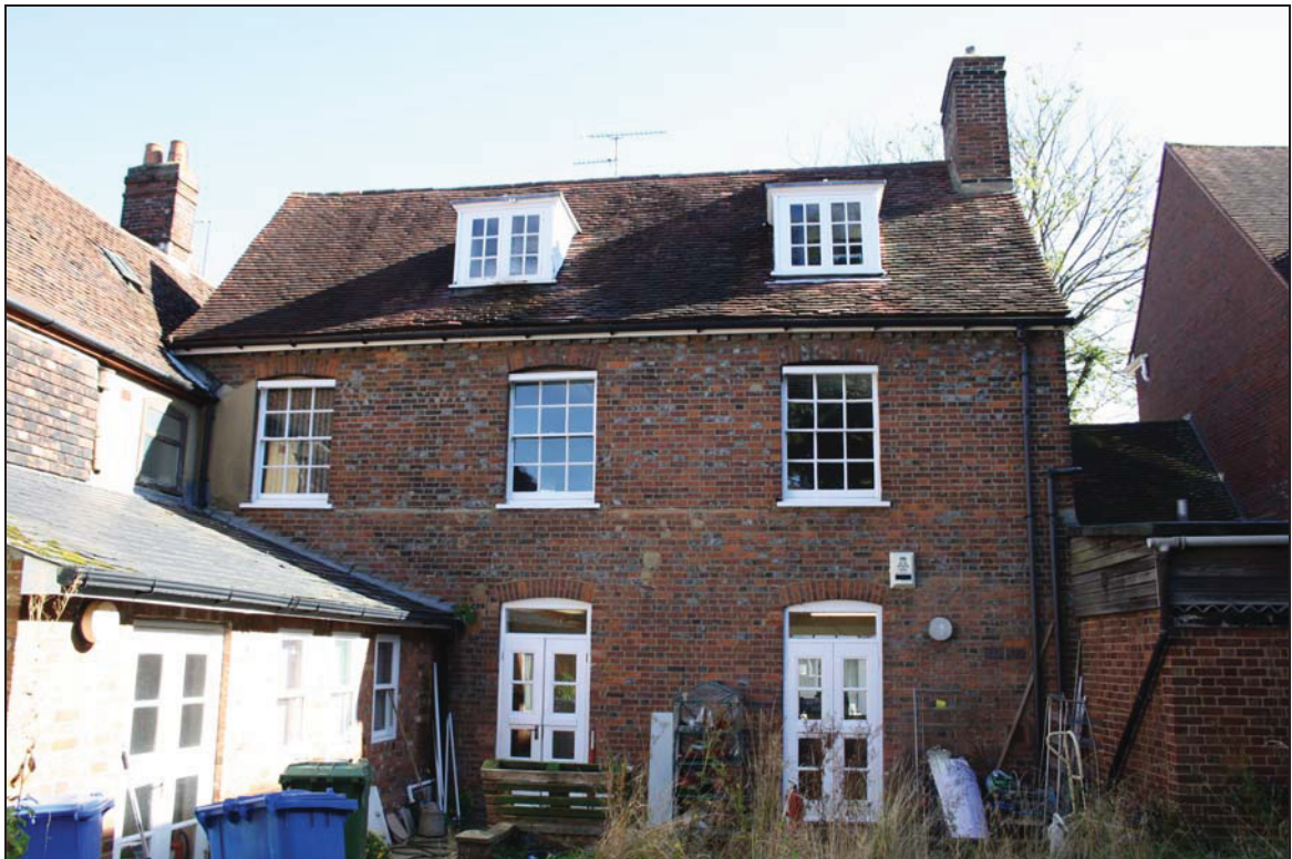
DP 28 Rear west elevation of the assessment building, taken from the west
