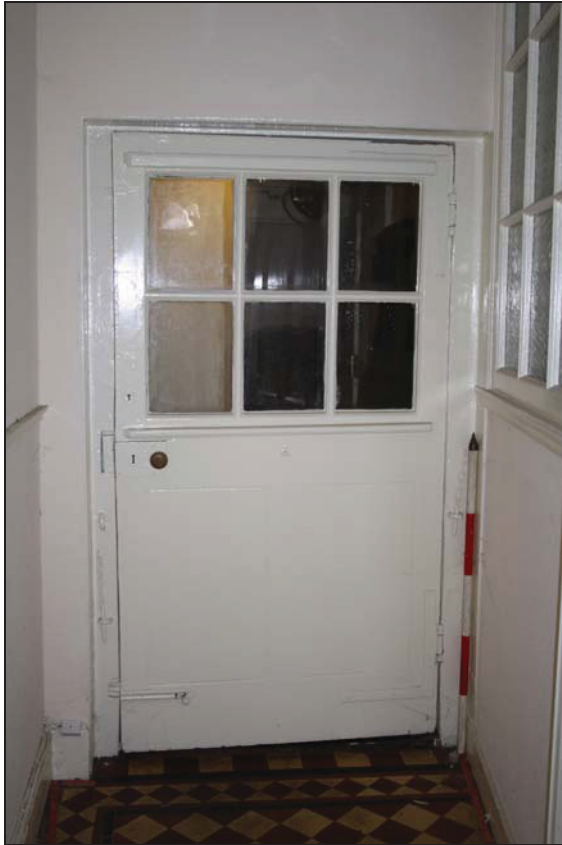
DP 10 Inner face of the original back door (GF02), taken from the east
