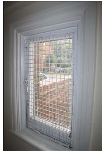
DP 16 Small single-light casement to the south-east range (GF02), taken from the north-west
