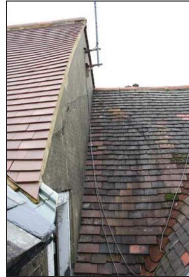
DP 8 Detail showing junction of the two roofs over No. 127, taken from the south
