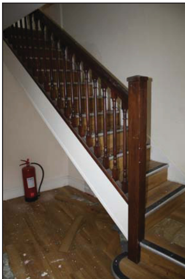
DP 17 Staircase in the south-east range (Room GF02), taken from the south-west
