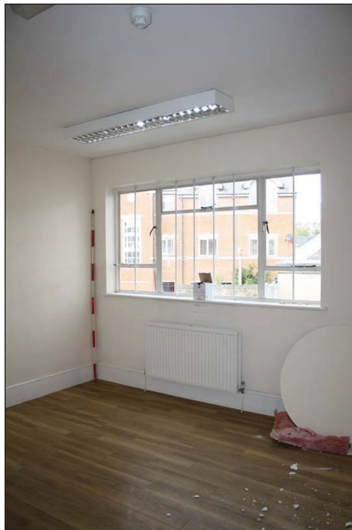
Plate 4 Room FF06 showing modern remodelling of the south-east range, taken from the east (DP 18)
