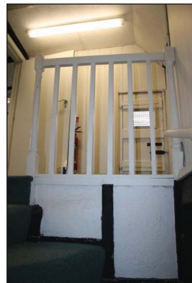
DP 12 Section of early balustrade at second floor level, taken from the west
