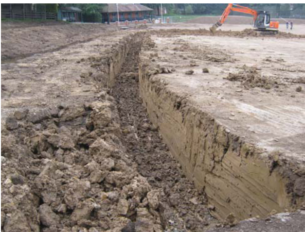
DP 9. Service trench in the eastern part of the site. Looking south-south-west.
