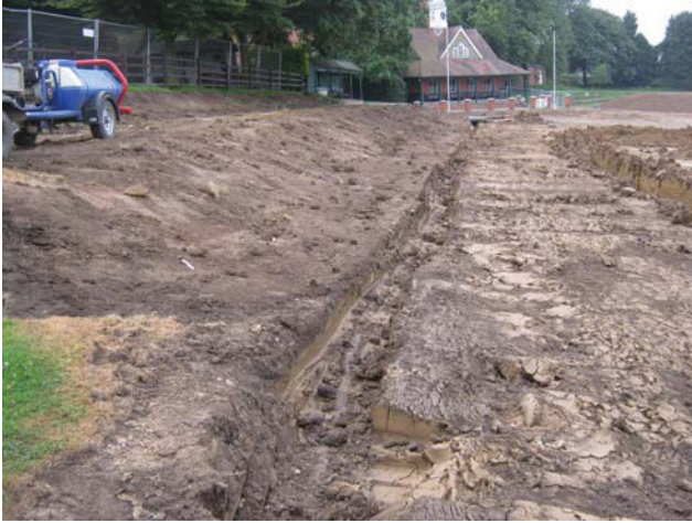
DP 7. Service trench in the eastern part of the site. Looking south-south-west.
