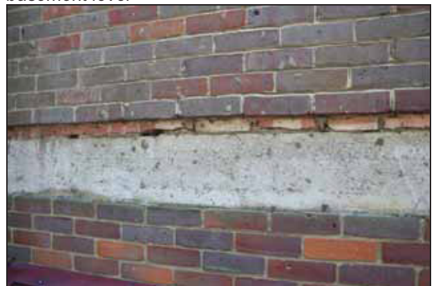
96 Exposed construction detail on the north side of Building A, taken from the north
