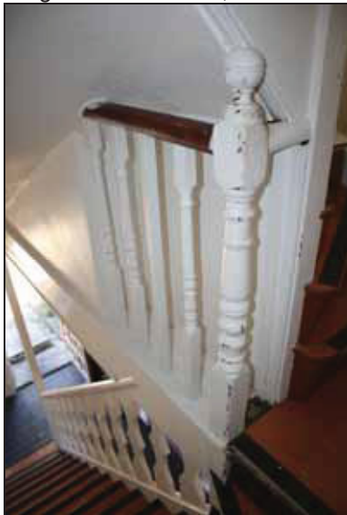
89 Detail of the secondary staircase in Building B, taken from the west
