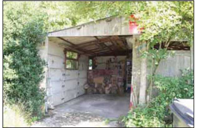
4 Pre-fabricated garage on the north side of the car park, taken from the south
