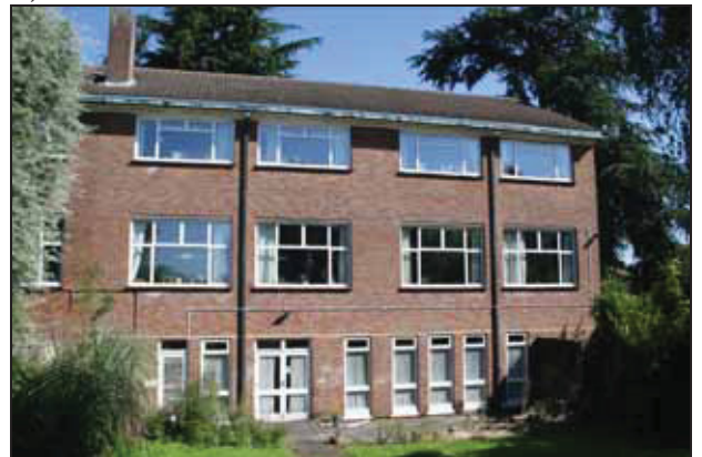
10 South elevation of Building C at the east end, taken from the south
