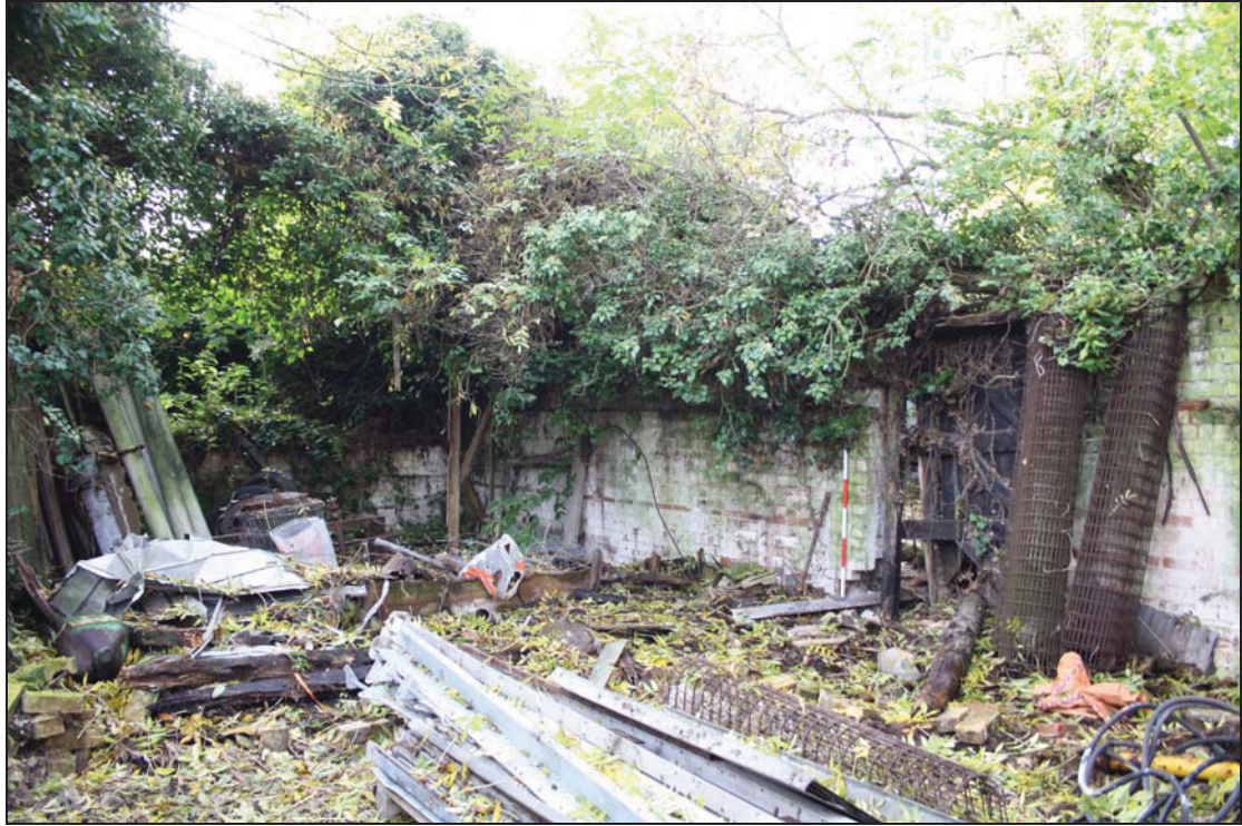
Plate 17 Surviving outer brick walls on the west side of Range 4, taken from the north-east (DP 55)
