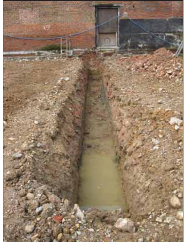
8 Footing trench to the south wall of the northern extension. Looking west.
