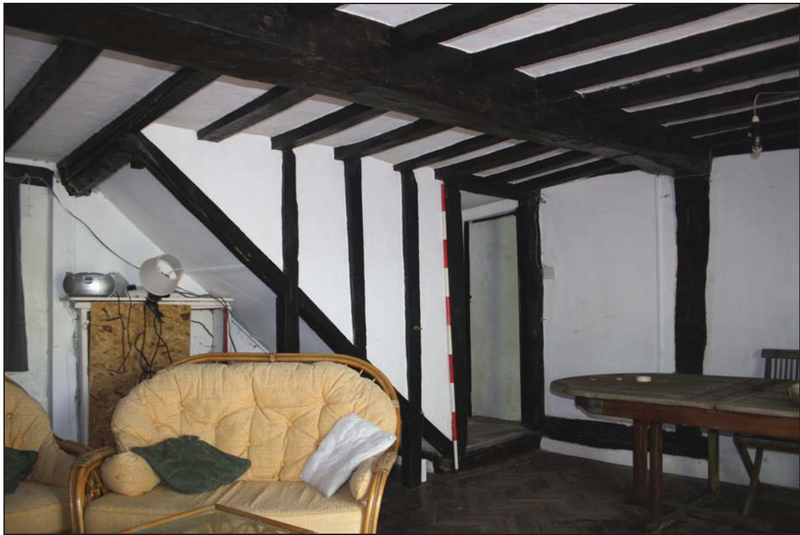
Plate 5 North-west area of Room GF01 showing enclosed staircase, taken from the south-east (DP 14)
