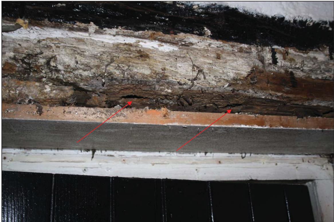
Plate 3 Detail of the formerly external north wall of the house from within Room GF04 showing wattle holes in the mid-rail (indicated), taken from the north-east (DP 21)
