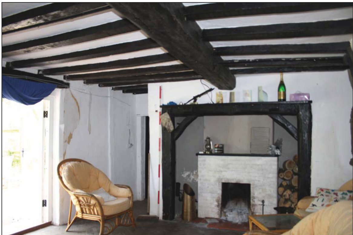
Plate 4 South side of Room GF01 showing inglenook fireplace, taken from the north (DP 15)
