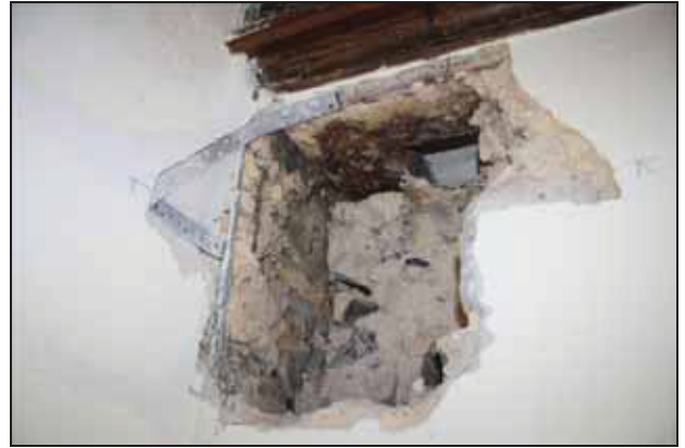
DP 116 Floor socket 4 on the north side of the chancel during the planned works, taken from the south-east
