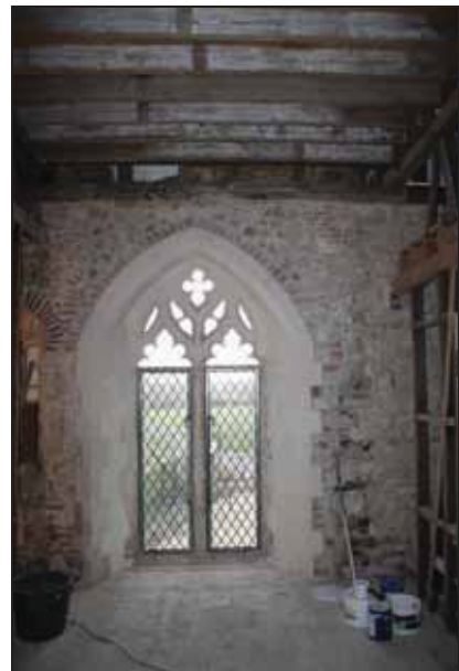
DP 108 South side of the nave (FF03) during planned works, taken from the north
