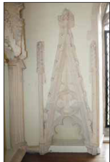
DP 48 Hood of the piscina on the south side of Room FF01, taken from the north
