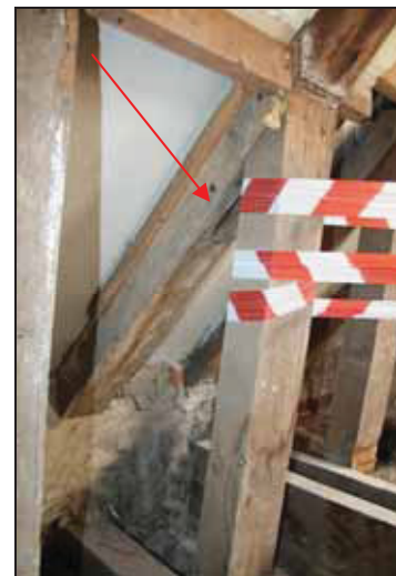
DP 90 North side of the nave roof showing replacement ashlar piece with empty mortice for the original (indicated), taken from the south-west
