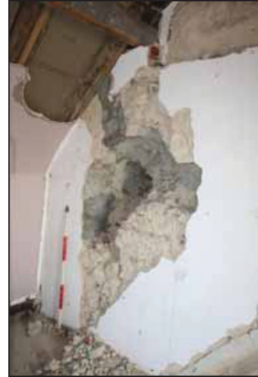
DP 86 View of the north side of the chancel arch during piercing of the northern doorway, taken from the south-west
