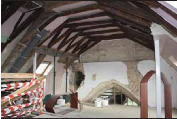
DP 103 General view of the nave at upper level during the planned works, taken from the west
