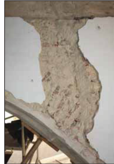
DP 88 Area of repair on the south side of the chancel arch showing brick repairs, taken from the west
