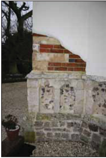
DP 7 Detail of the south-west buttress of the tower, taken from the south-east
