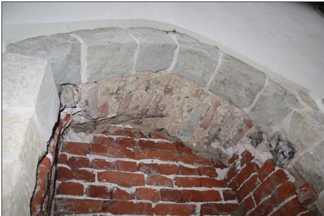
Plate 4 Arch soffit on the blocked doorway on the north side of the chancel, taken from north (DP 13)
