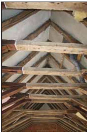
DP 89 View of the apex of the roof over the nave, taken from the east
