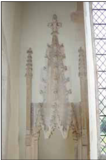
DP 45 Hood of image niche on the east side of Room FF01, taken from the west
