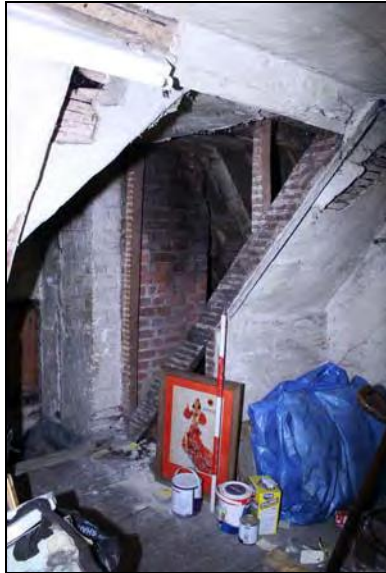
43 North side of Room SF01 at the top of the staircase flanking the chimney stack, taken from the south- west
