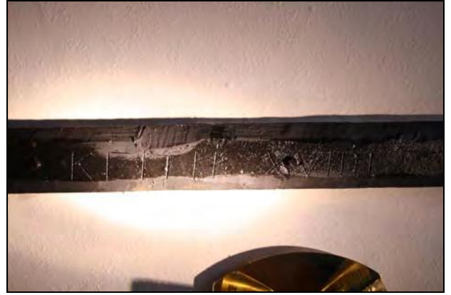
20 Graffiti on a ceiling joist in Room GF02, taken from the west
