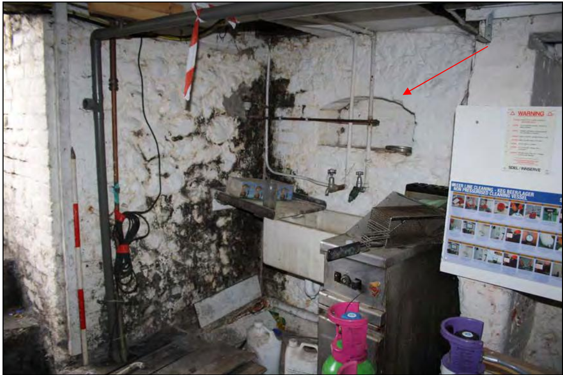
Plate 11 North-west corner of Room BF showing flint construction and original niche (indicated), taken from the south-east (17)
