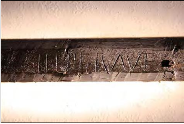
19 Graffiti on a ceiling joist in Room GF02, taken from the west
