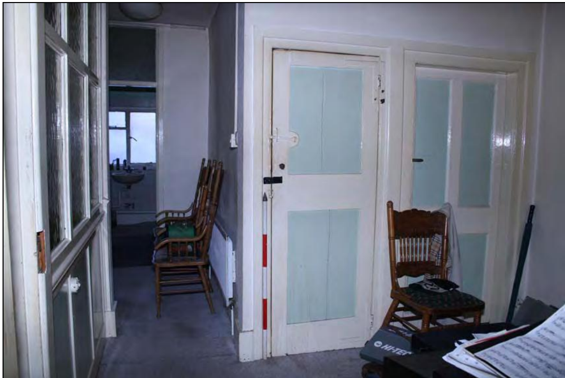
Plate 6 East side of Room FF01 with surviving original door in the centre, taken from the west (31)
