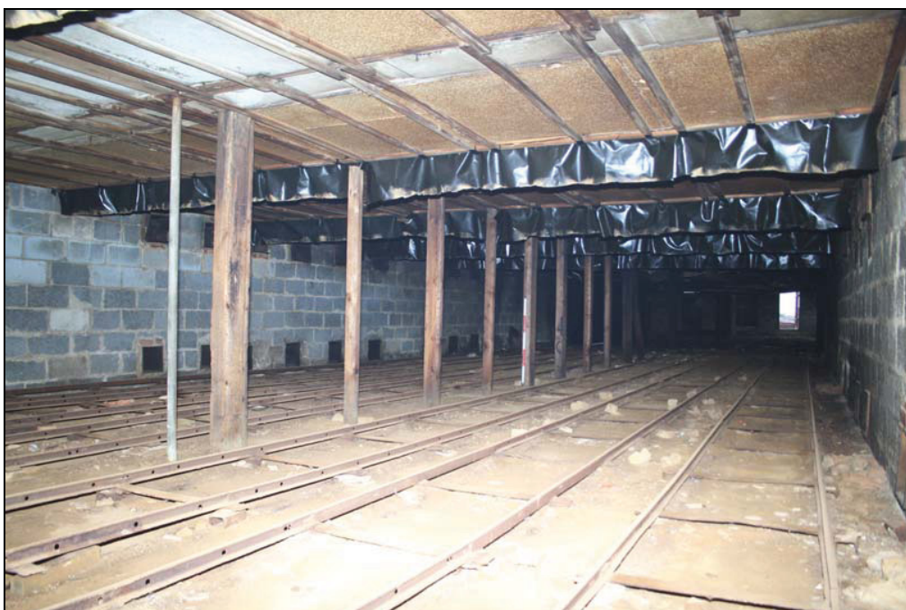
Plate 4 Central section of Building 1 lined with trackways, taken from the north-west (DP 58)
