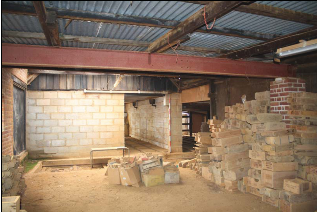
Plate 9 Stacked brick moulds, north-east extension to Building 3, taken from the north-east (DP 79)
