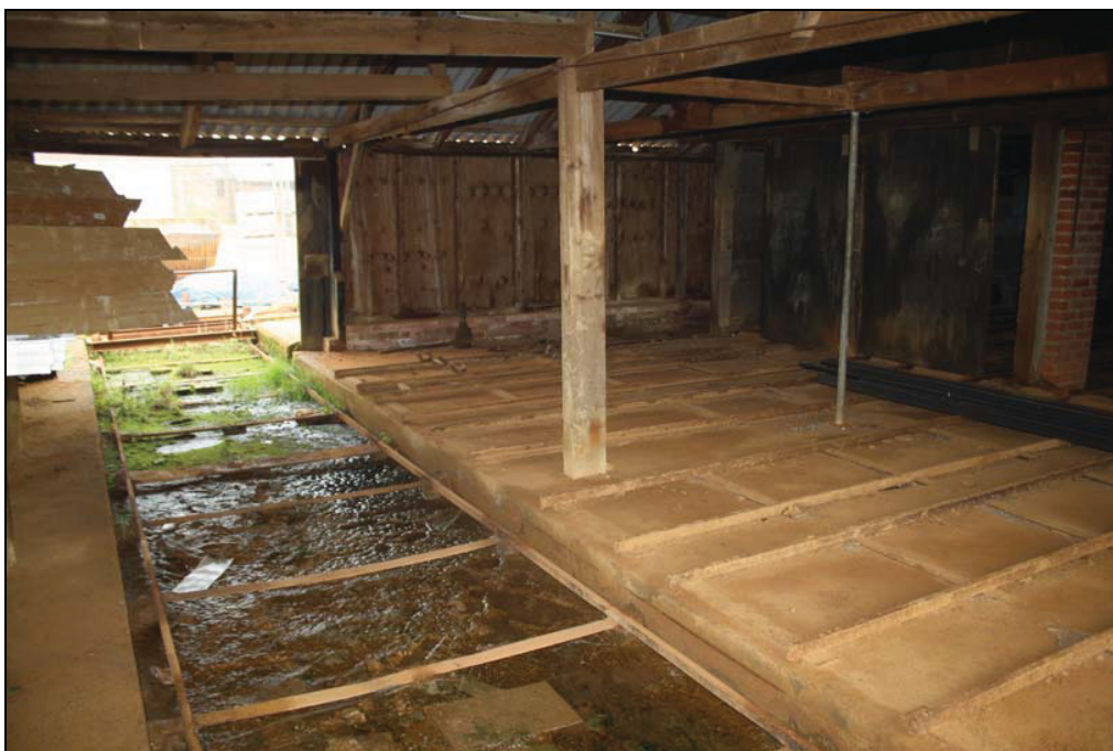
Plate 3 Series of trackways with a lateral track and surviving moveable trolley, north end of Building 1, taken from the north-west (DP 54)
