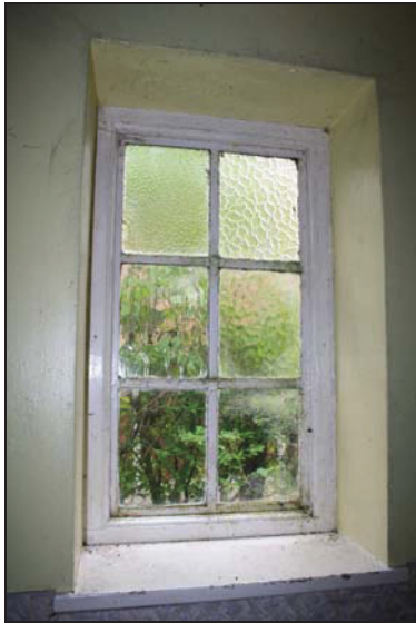
DP 13 Fixed window in the entrance porch (church), taken from the south-west
