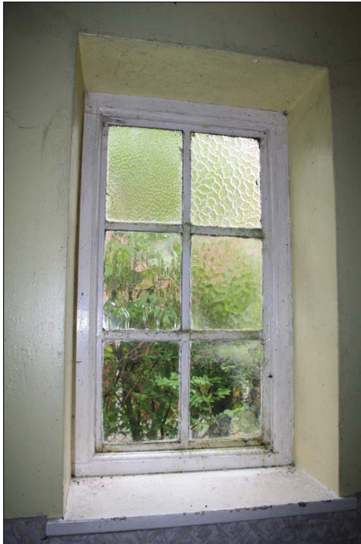
Plate 3 Fixed window in the entrance porch (church), taken from the south-west (DP 13)
