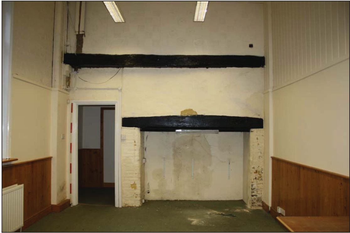
Plate 5 Former west end of the truncated bays of Range 1 from within Range 2, taken from the east (DP 19)
