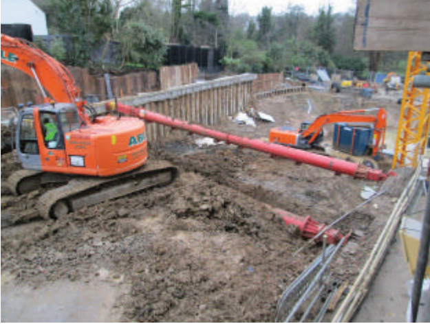
DP 19. Eastern and central part of the site during the ground reduction. Looking south-west.
