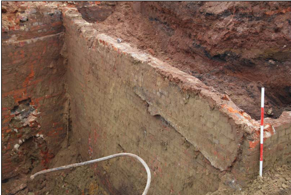
Plate 8 The remains of the roof line along the eastern retaining wall, taken from the south-west (DP 60)
