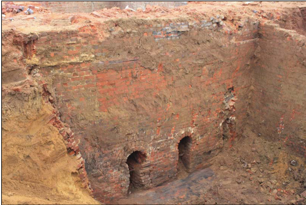
Plate 4 External archways along the south wall of the kiln, taken from the south-west (DP 61)
