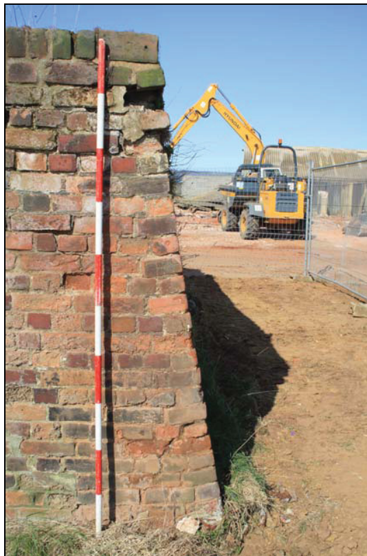
Plate 2 Battered northern end of eastern elevation, taken from the east (DP 5)
