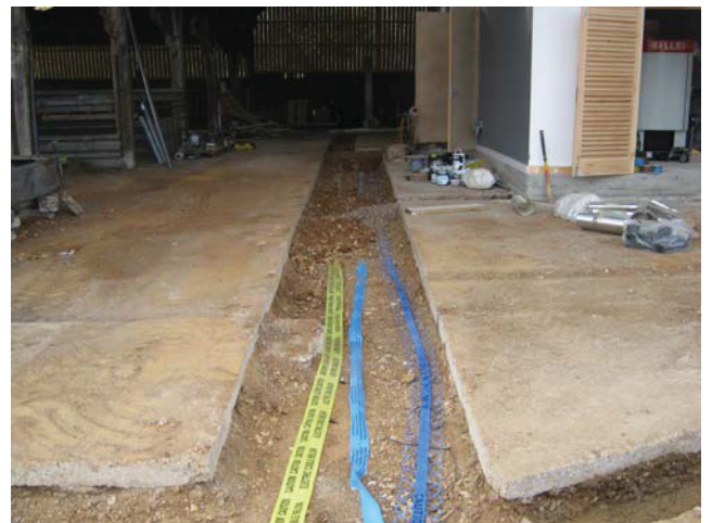
DP 6. Backfilled trenches inside barn next to installed biomass boiler. Looking north-west.
