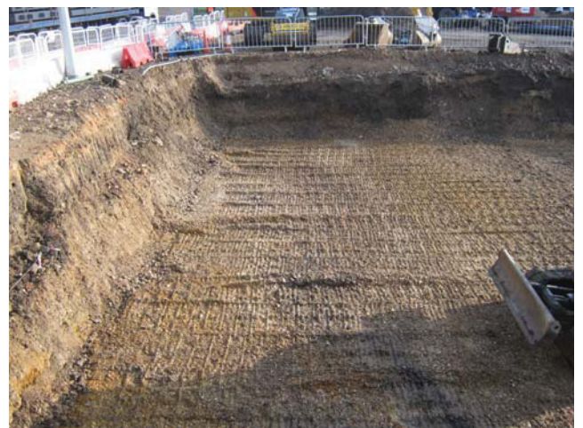
DP 12. Attenuation tank No 2. Looking north-east.
