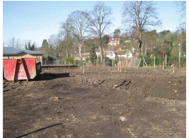
DP 2. Ground reduction area within the northern part of the site. Looking north-west.
