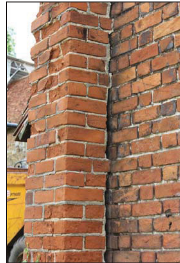
DP 10 Detail of the later attached chimney stack on the west elevation of the lean-to, taken from the south-west
