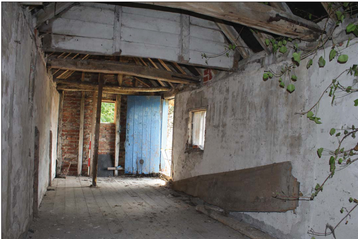
Plate 6 Upper floor of the assessment structure (Room FF01), taken from the west (DP38)
