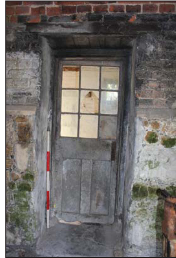
DP 26 Doorway on the south side of Room GF03 leading to the main range, taken from the north
