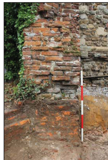
DP 60 Section of the pre-existing brick pier with brickwork below exposed during ground reduction, taken from the west
