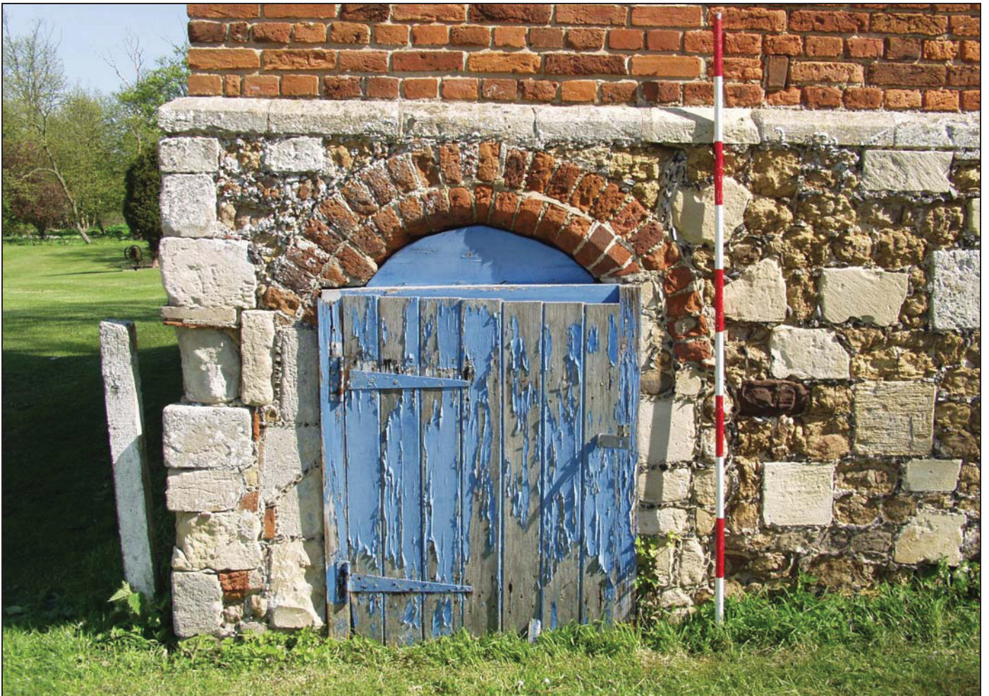
Plate 2 Arch on the south elevation (west end), taken from the south (DP03)
