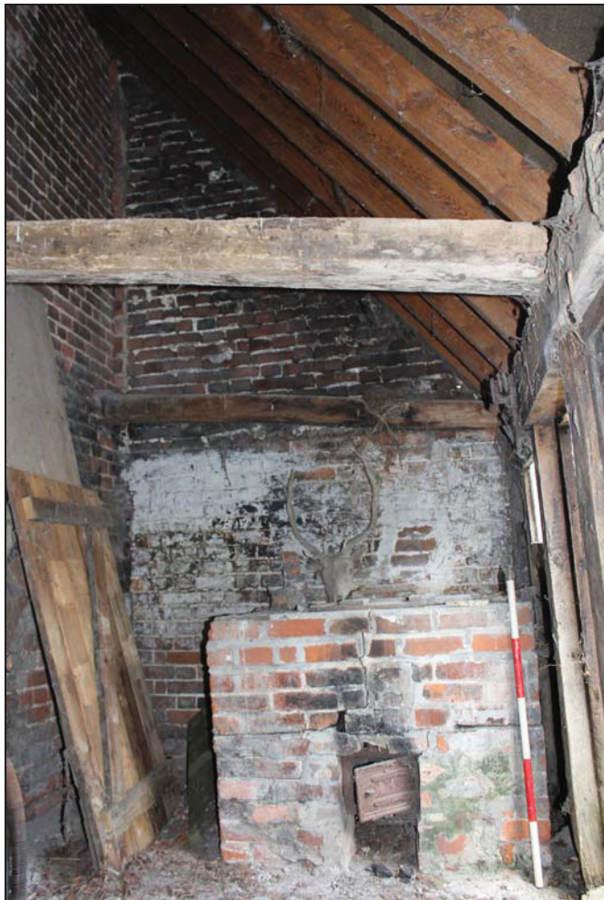
Plate 5 West end of Room GF03 in the lean-to, taken from the east (DP29)
