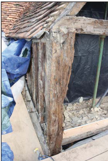
DP 51 Exposed timber-framing on the west elevation of the rear range, taken from the south during monitoring
