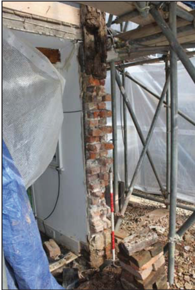
DP 59 East end of the south gable at ground floor level after removal of later brickwork, taken from the south-west during monitoring
