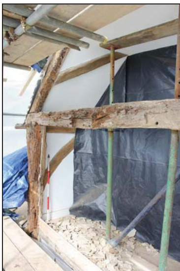
DP 45 Surviving principal timbers at first floor level, taken from the south-east during monitoring
