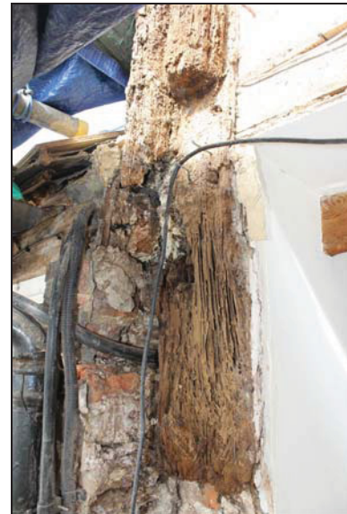
DP 62 Truncated south-west corner post showing exposed mortice for the lost mid-rail, taken from the south- east during monitoring
