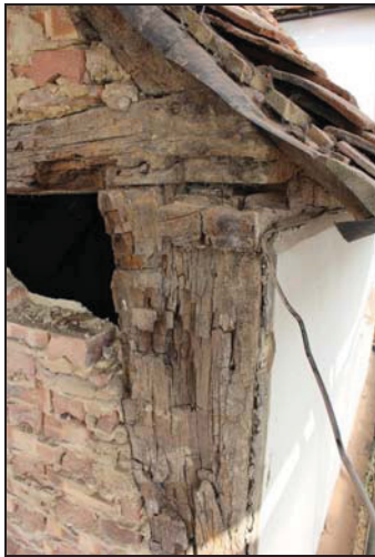
DP 43 Framing arrangement at the head of the south-east corner post showing chamfered wall-plate (partially lost), taken from the south during monitoring
