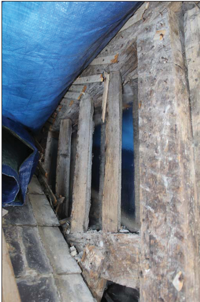
Plate 7 Original mullion window on the west elevation exposed after the removal of lath and plasterwork, taken from the south-west during monitoring (DP 59)
