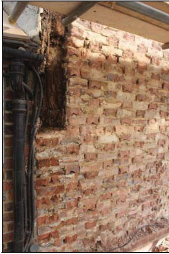
DP 41 Truncated and degraded south-west corner post, taken from the south-west during monitoring
