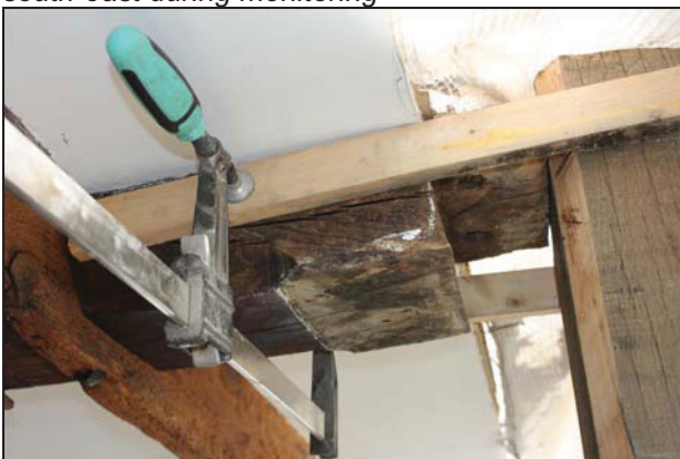
DP 63 South end of the bridging joist in the sitting room showing pegged tenon for the lost mid-rail, taken from the west during monitoring
