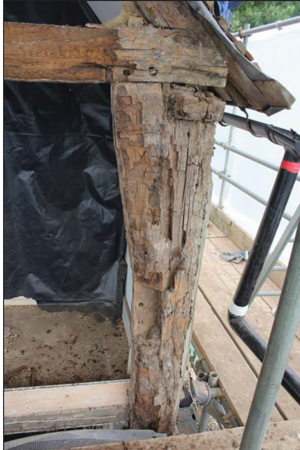
Plate 5 South-east corner post showing exposed brace mortise, taken from the south during monitoring (DP 48)
