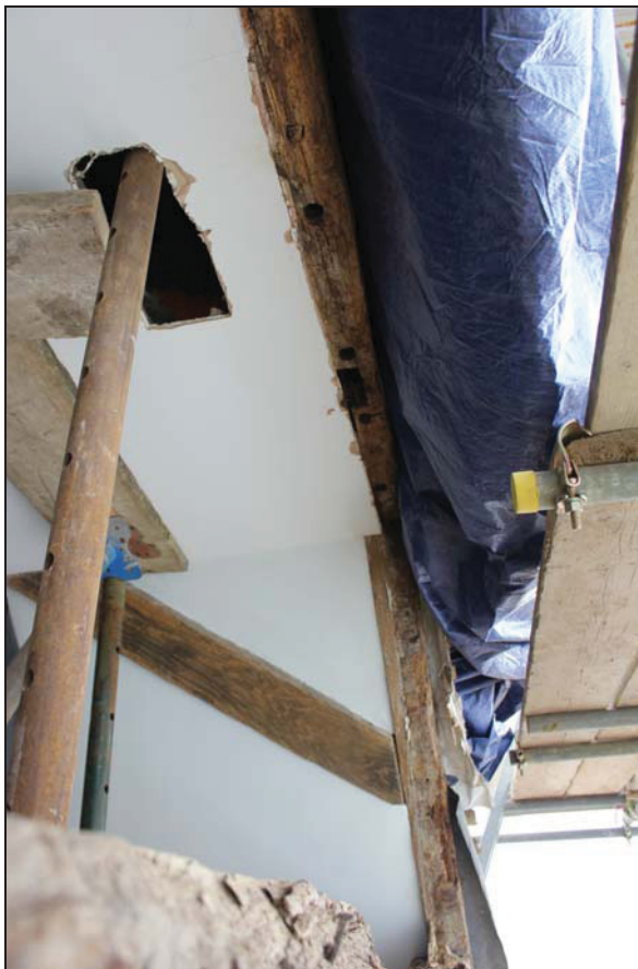
Plate 6 View of the collar soffit showing wattle stave holes, taken from the west during monitoring (DP 50)
