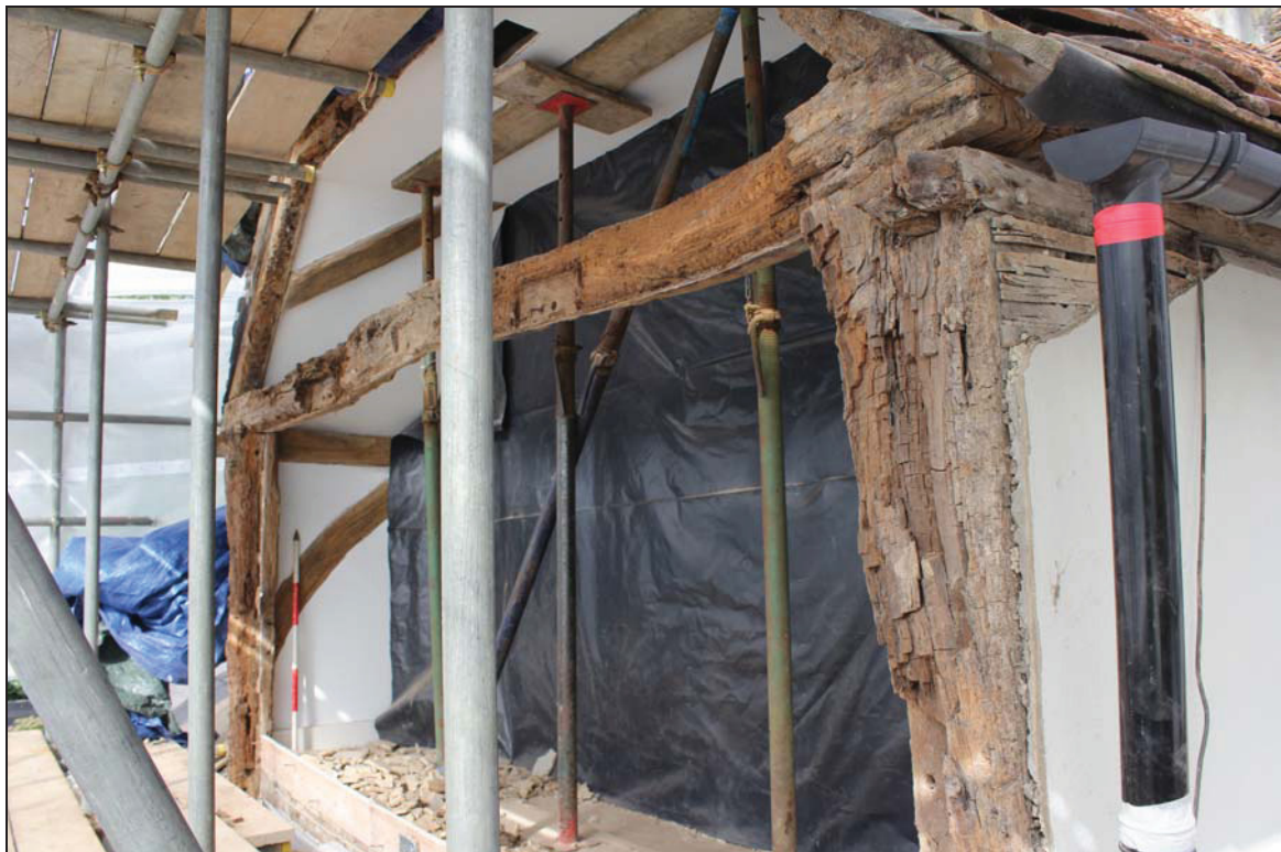
Plate 4 Surviving principal timbers at first floor level, taken from the south-east during monitoring (DP 44)
