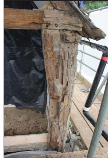
DP 48 South-east corner post showing exposed brace mortice, taken from the south during monitoring
