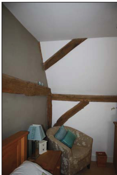
DP 23 Detail of the timber-framing in the south-west corner (Bedroom 3), taken from the east
