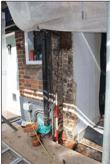
DP 61 West end of the south gable at ground floor level after removal of later brickwork, taken from the south-east during monitoring
