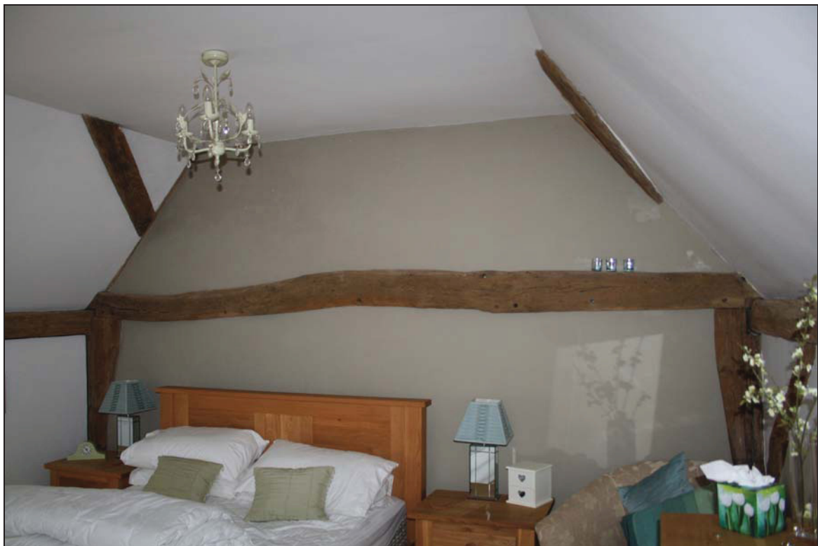
Plate 8 First floor room of the rear wing (Bedroom 3) showing the gable end, taken from the north (DP 21)
