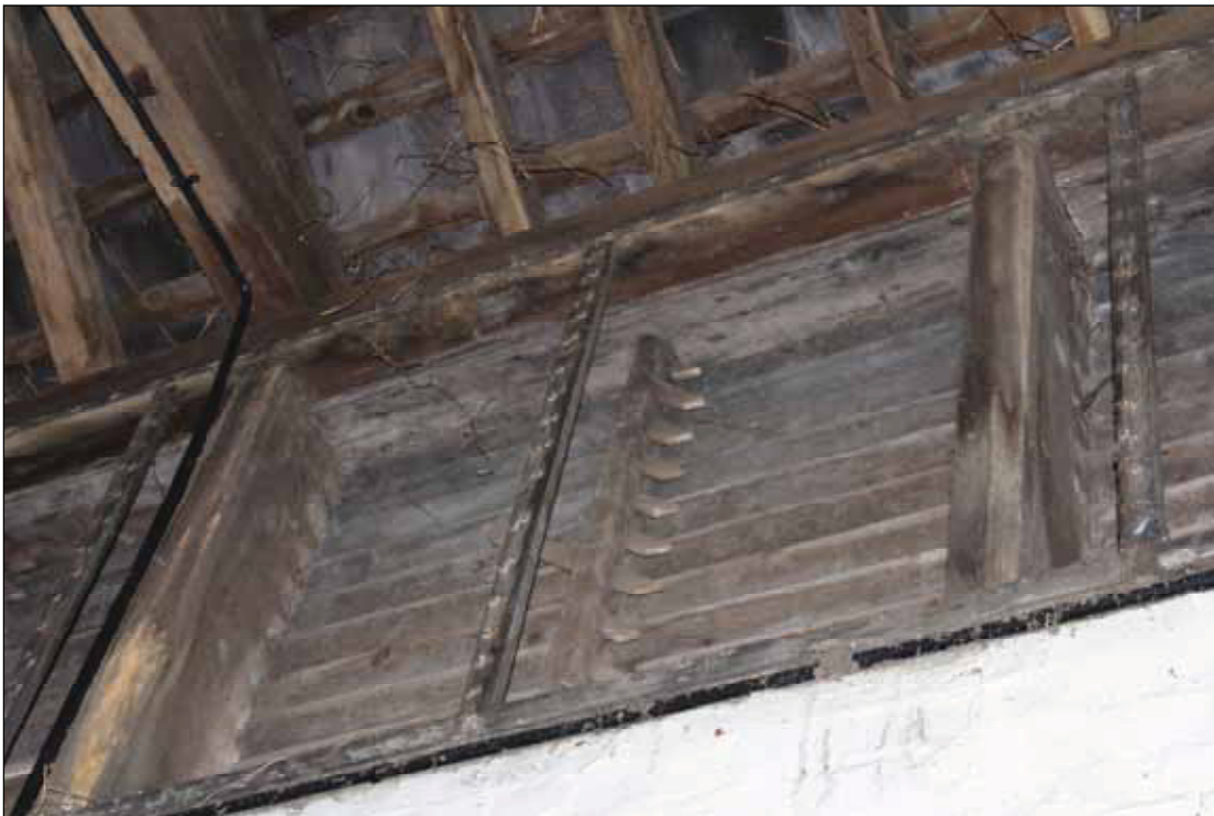
DP 24 Opening mechanism for ventilation louvres, taken from the south-east
