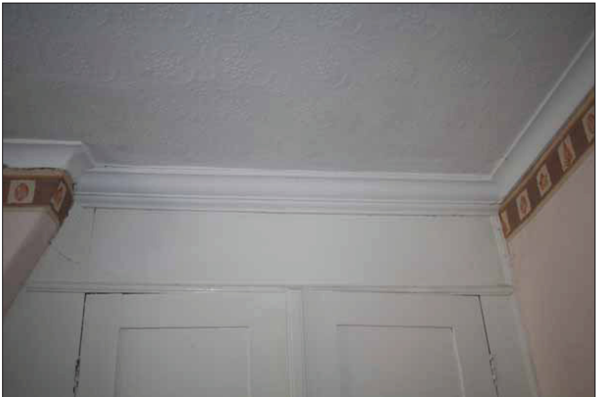
Plate 8 Surviving stretch of 18th century cornice in the north range (first floor), taken from the west (DP 74)
