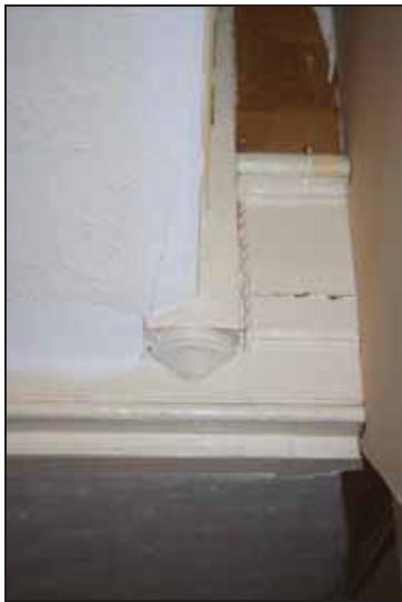
DP 51 Staircase finial in the stair hall of the north range (ground floor), taken from the north
