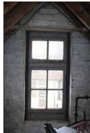
DP 72 Window on the east side of the south range of Outbuilding 2 (first floor), taken from the west
