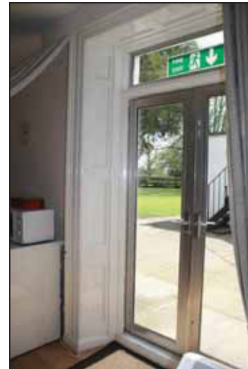
DP 70 Entrance on the south side of the staff lounge in the north range (ground floor) showing panelled reveals, taken from the north-west
