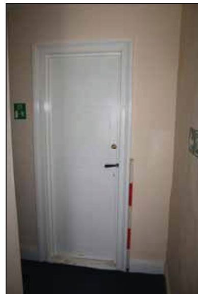
DP 54 Door to the closet in the north range (first floor), taken from the south
