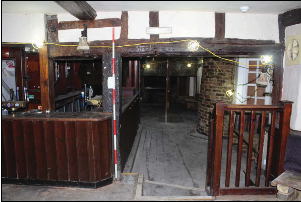
Plate 7 Junction between the medieval core and 17 th century extension, GF02, taken from the south (DP 26)
