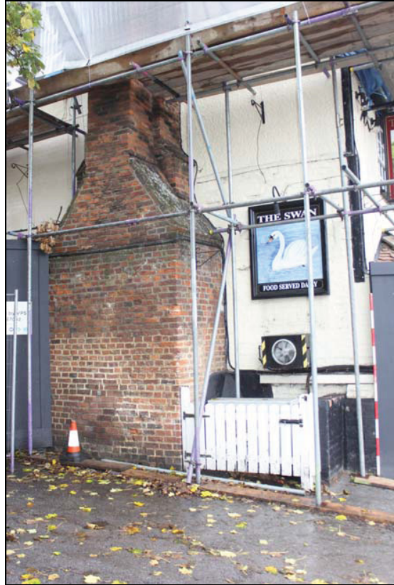
Plate 5 Lower portions of the chimney stack, south elevation, taken from the south-east (DP 3)
