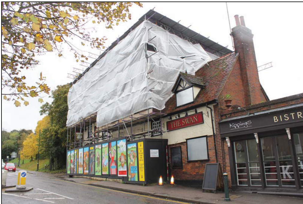
Plate 4 The Swan, (post-fire) taken from the north-east (DP 4)
